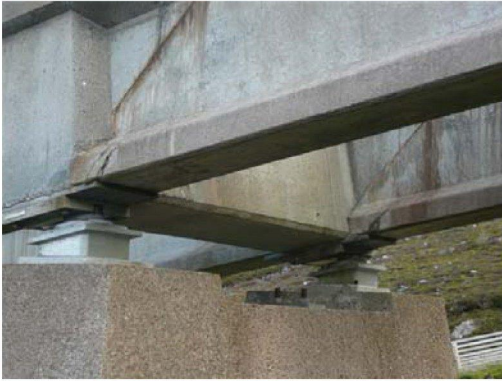
Photo [14] Diagonal cracks through the lower flange of the precast beam bearings.
