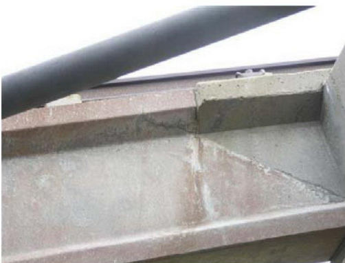
Photo [16] Flange fracture also seen at top of beams. This was less often.
