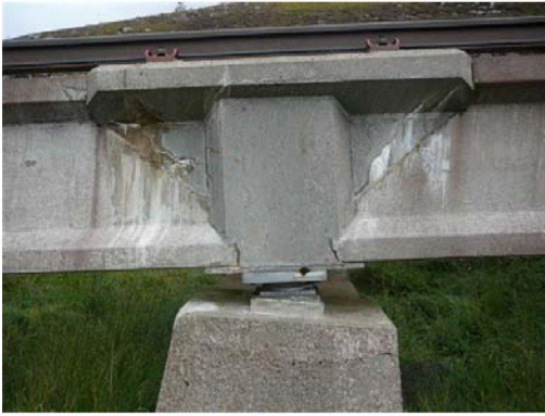
Photo [12] Pier 8, one of the poorer insitu infills. Showing joints opening between Insitu and precast plus cracking within the mass of the Insitu, both inclined and near vertical.
