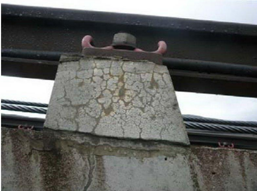
Photo [1] Typical grout plinth, exhibiting crazing, but stable
