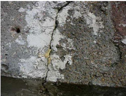
Photo [11] Pier 56 crack near top of flange as train passes. Estimate increase in crack width = 1.0mm.
