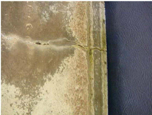
Photo [6] View of crack on typical mid-span underside of beam.
