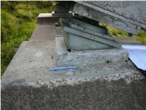
Photo [20] Showing deterioration of bearing plate grout.
