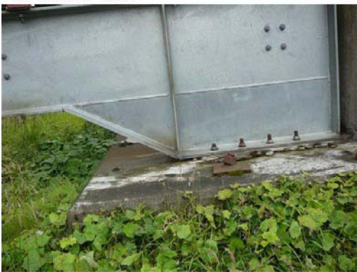
Photo [21] Crumbling grout pack under steel beam at pier 0.
