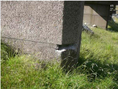
Photo [18] Significant chip out of pier shell.
