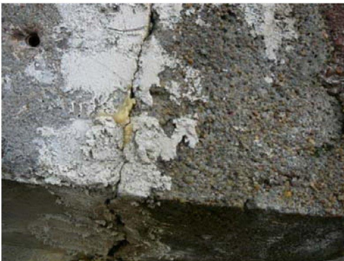
Photo [10] Pier 56 crack near top of flange unloaded.
