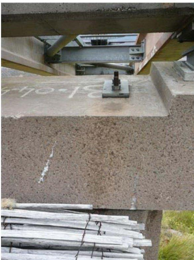
Photo [19] Pier 93. Crack rising up through pier crosshead and passing through bolt group. This was the only cross head where this was observed.
