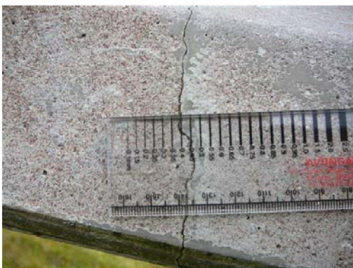
Photo [7] The above photographed crack as it appears on the side of the beam.
