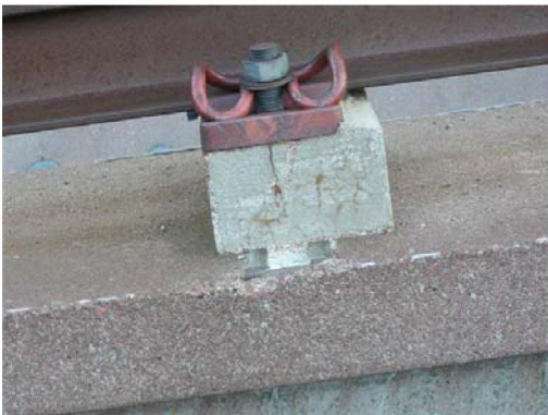
Photo [3] Grout plinth showing fracture. Regarded as stable at this time.
