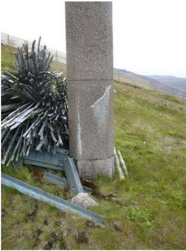
Photo [17] Main pier 91 showing cracks in shell.
