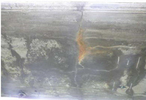
Photo [8] Crack at mid span of beam exhibiting rust staining.
