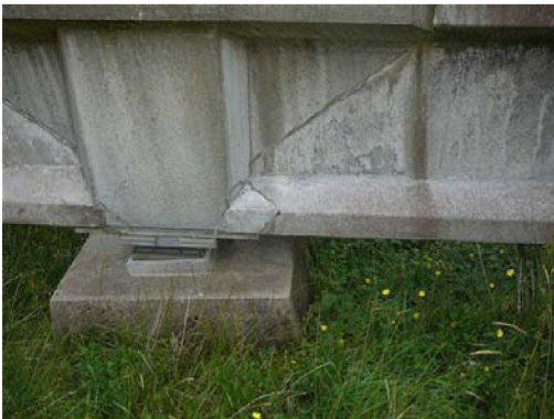
Photo [15] Showing bottom corner fracturing away.
