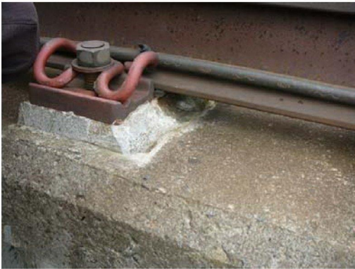
Photo [2] Typical case of a flake off one face of plinth. This regarded as stable.
