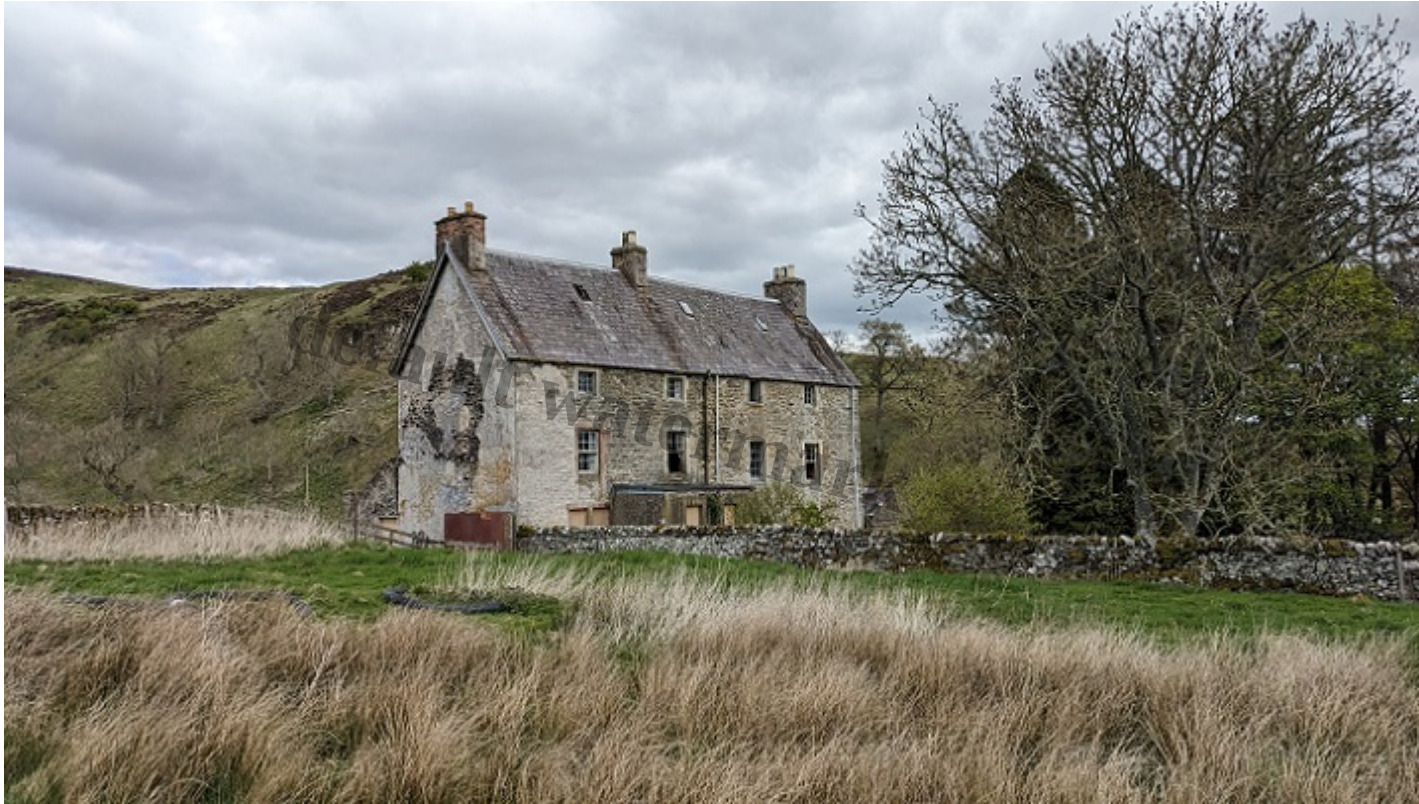
The B-listed farmhouse at Todrig, which has been allowed to fall into a state of disrepair. 15th May 2026
