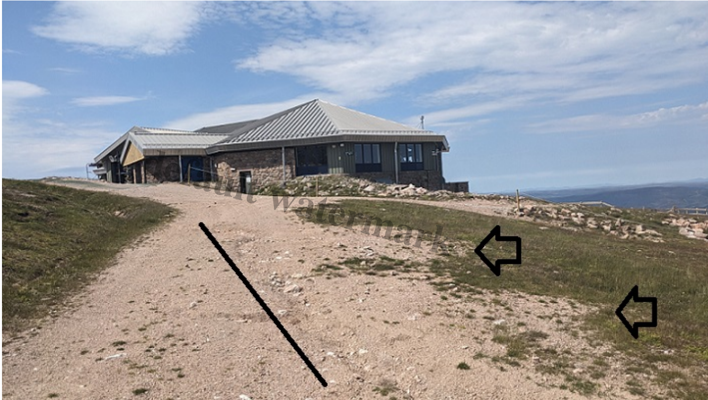
Track erosion by the Ptarmigan, with the black line indicating the current erosion channel and the black arrows areas where the track surfacing has washed out over vegetation. Photo 2025,
