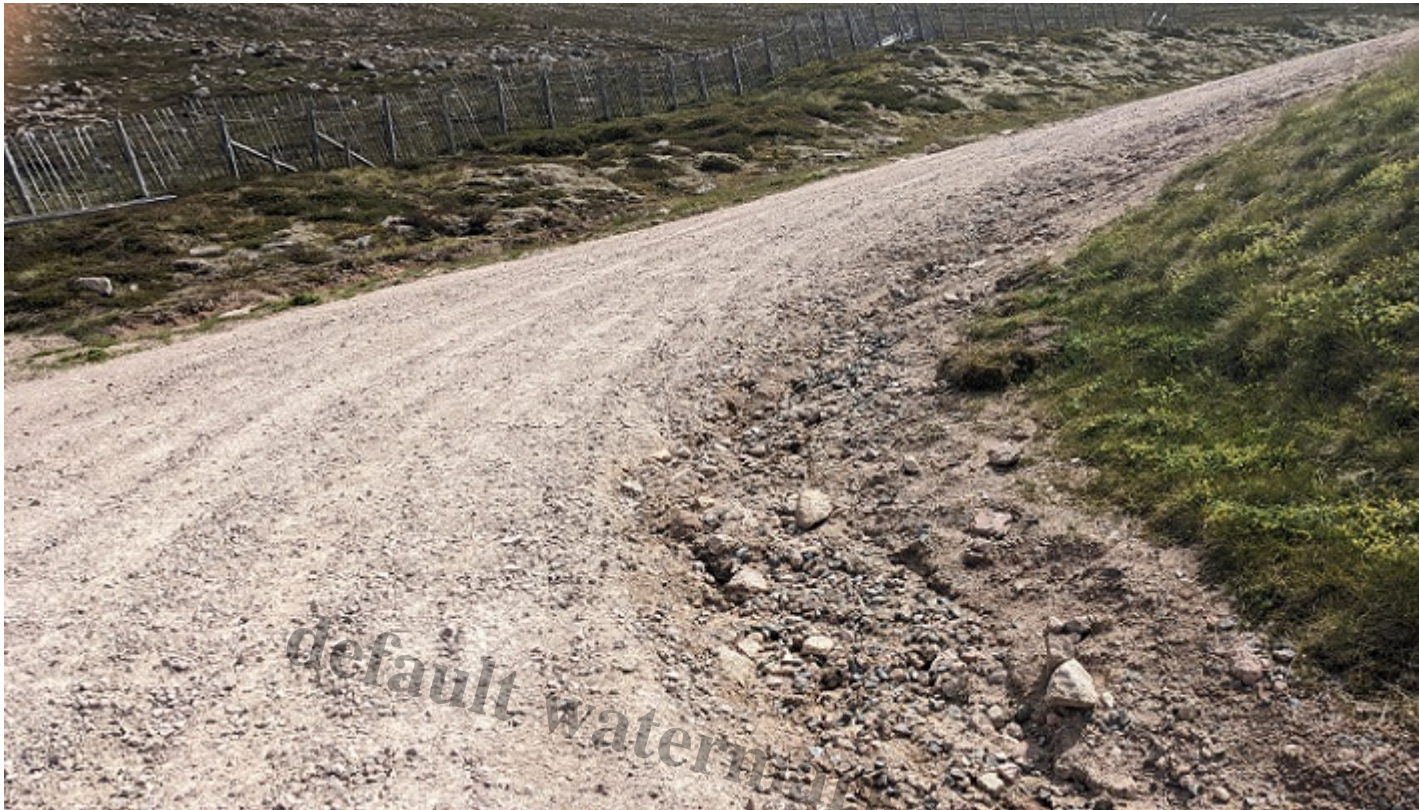
and the right. Erosion gully on opposite side of track to photo above
