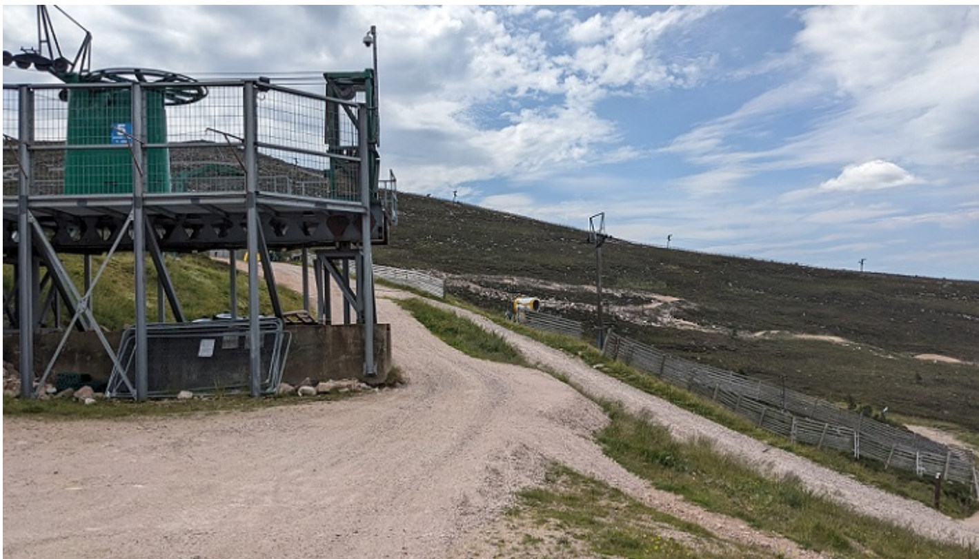
New surfacing of track at the Shieling poised to wash downhill July 2025
