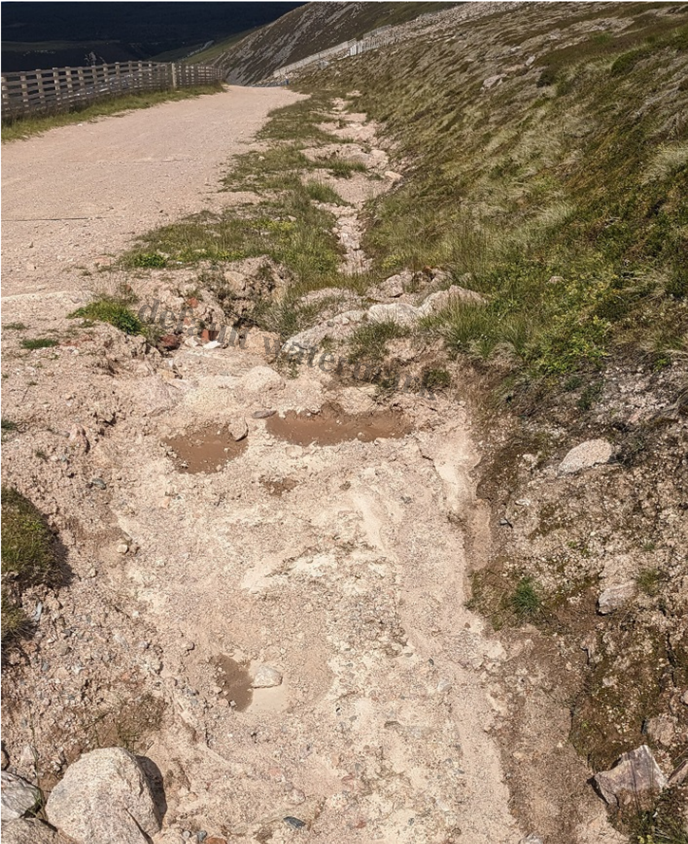
Note the different grades of material with the finest holding in the water and showing as damp patches. Photo July 2025.
