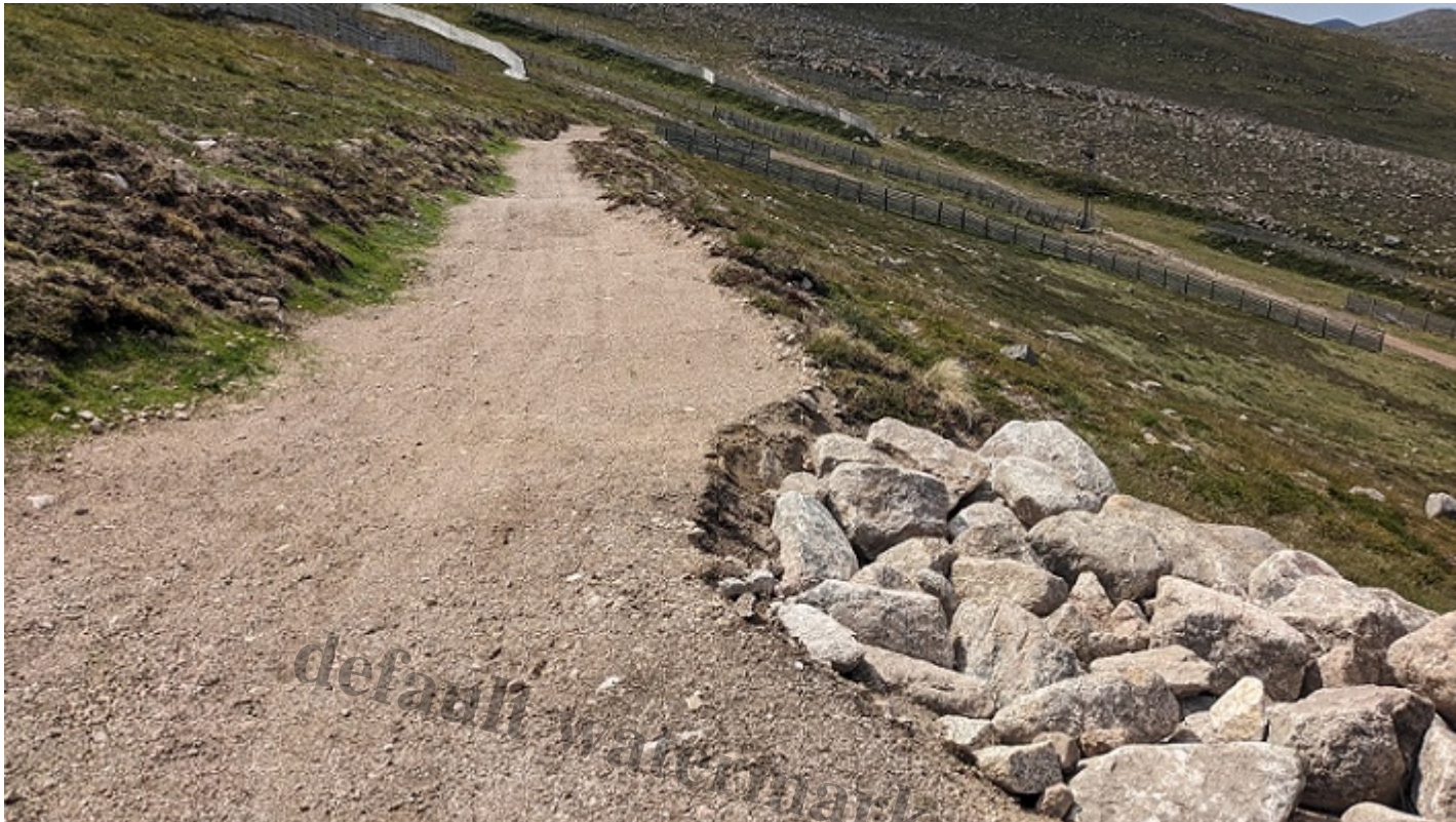
Collapse of new section of kart track (which incidentally never appears to have had planning permission) July 2025 illustrating how erosive forces punish poor design
