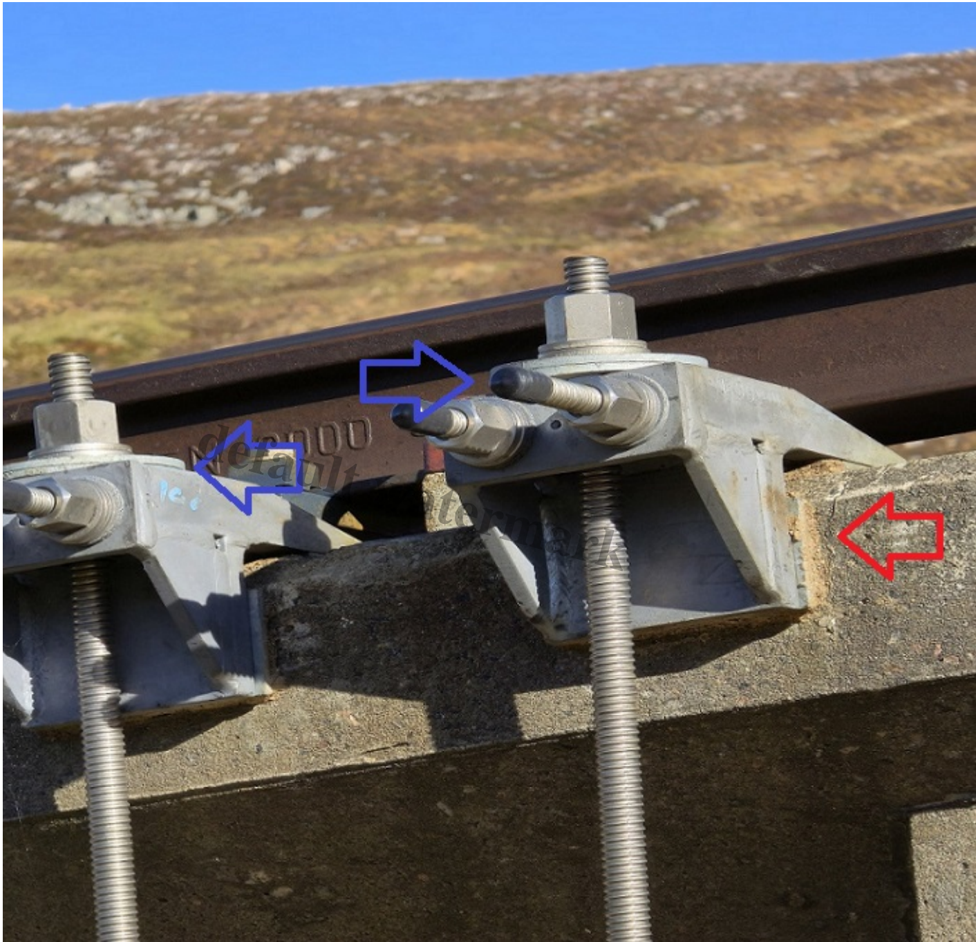
Besides too many washers there also appear to be a crack in the top flange, red arrow (Photo 4/706).
