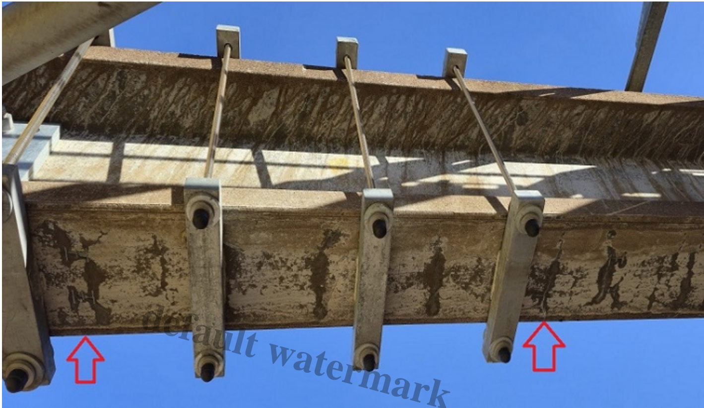
Left arrow shows exposed metal rebar, right a crack (Photo 8a/404)
