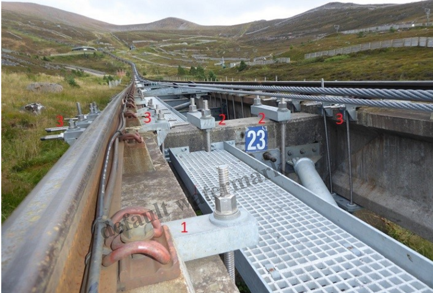
The figure one shows the position of the brackets round the beams referred to under Issue 2 below
