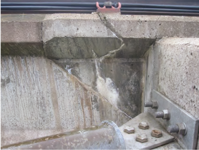
Cracking at Pier 9, where the spanner was found, but before the brackets were fitted. Photo courtesy of the COWI report Dec 2018.
