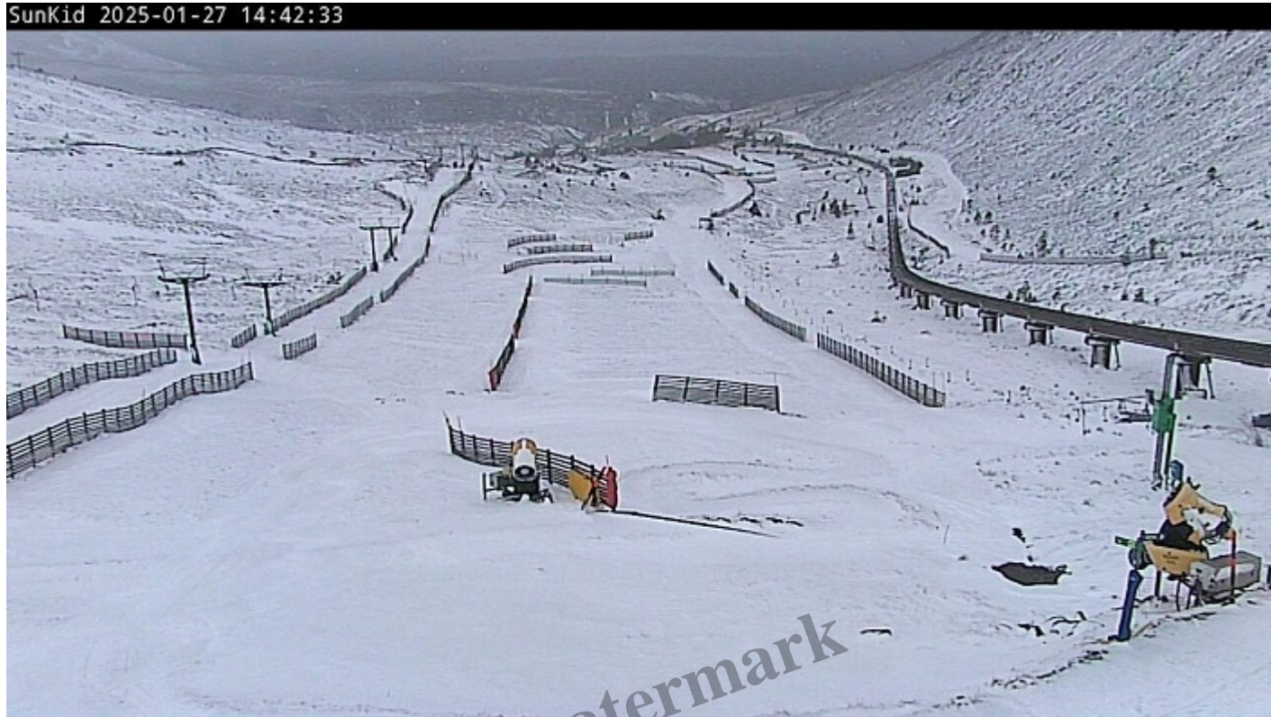
Same day, two snow cannon not working above the sunkid rope tow, installed to create a new beginners area. Photo credit CM(S)L webcam
