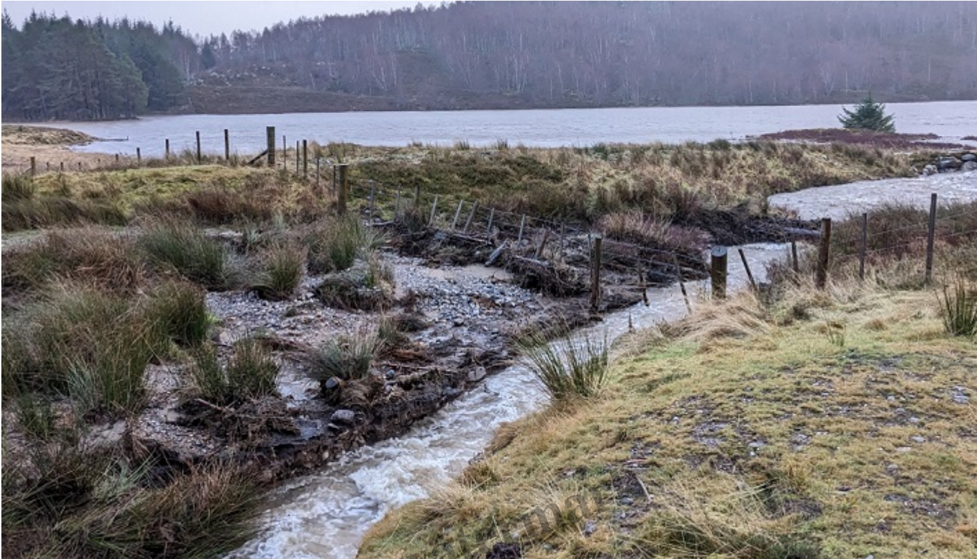
The outflow of the overflow channel viewed from the eroding section of bank. Note the difference between the still half bare bank in the foreground with the heavily vegetated bank beyond
