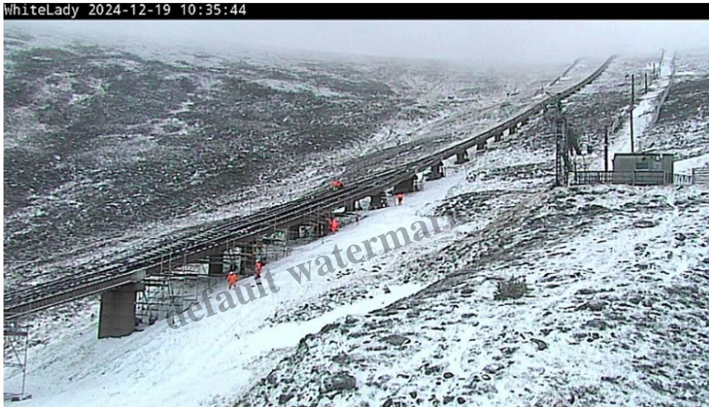
Funicular passing loop with scaffolding and workers 19th December – Cairngorm Mountain Scotland Ltd webcam
