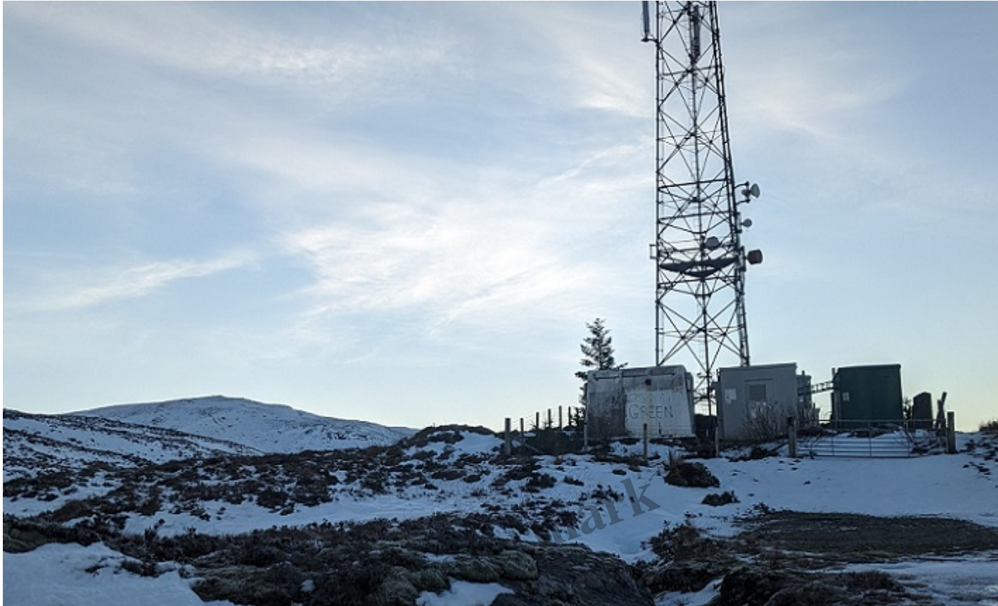
View of telecommunications tower with Meall Buidhe behind. Note the trees within the enclosure, including willow by the gate and in front of the central grey building and young sitka in the left hand corner.
