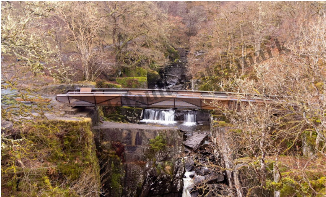
Variations of the size of the holes in the side panels as well as their colour affect how the bridge looks from the air. Clever! But who will see this? Photo credit IABSE awards.
