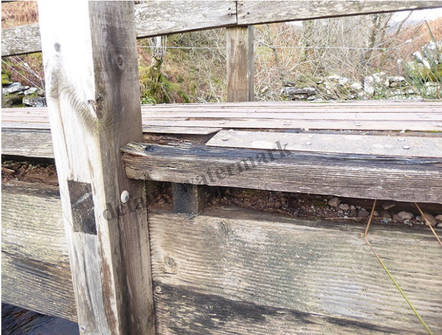
Detail of bridge showing rotten wood
