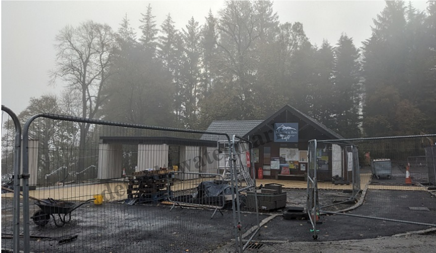
Photo of cafe area, with new shelter on left, still cordoned off from the car park with Heras fencing 28th October
