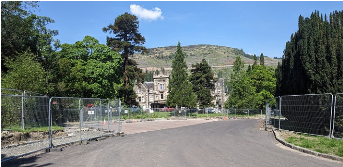
View of new campervan parking area in May with the unfinished pavement on left
