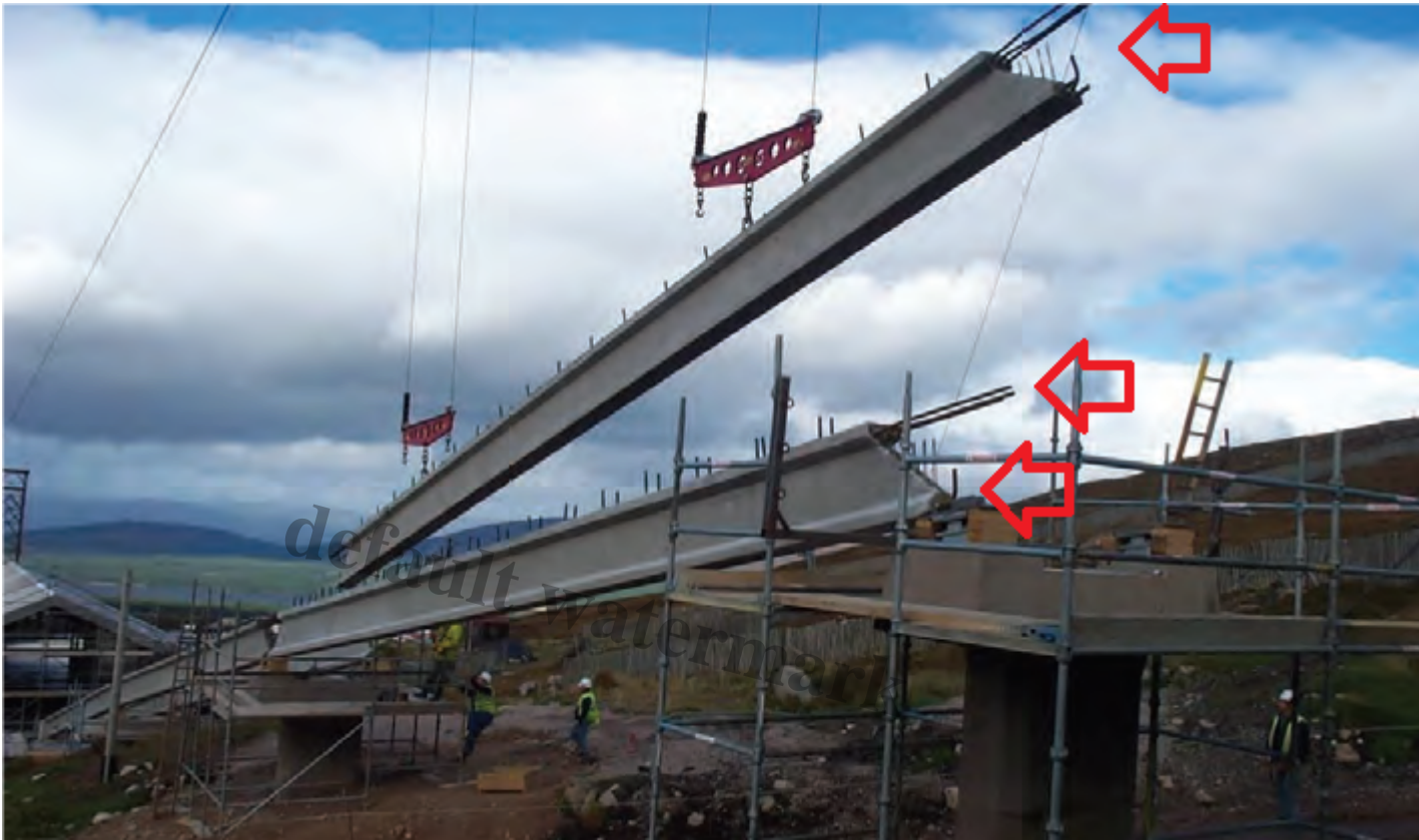
Figure 3-1 Precast beam installation from Cowi Report showing protruding rebars
