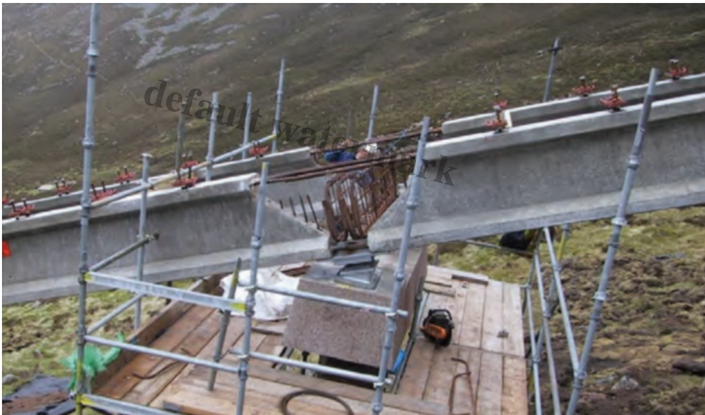
The insitu joint during construction showing the rebars and how the bottom ends of the beams rests on a small metal plate. Photo credit Cowi Report 2018
