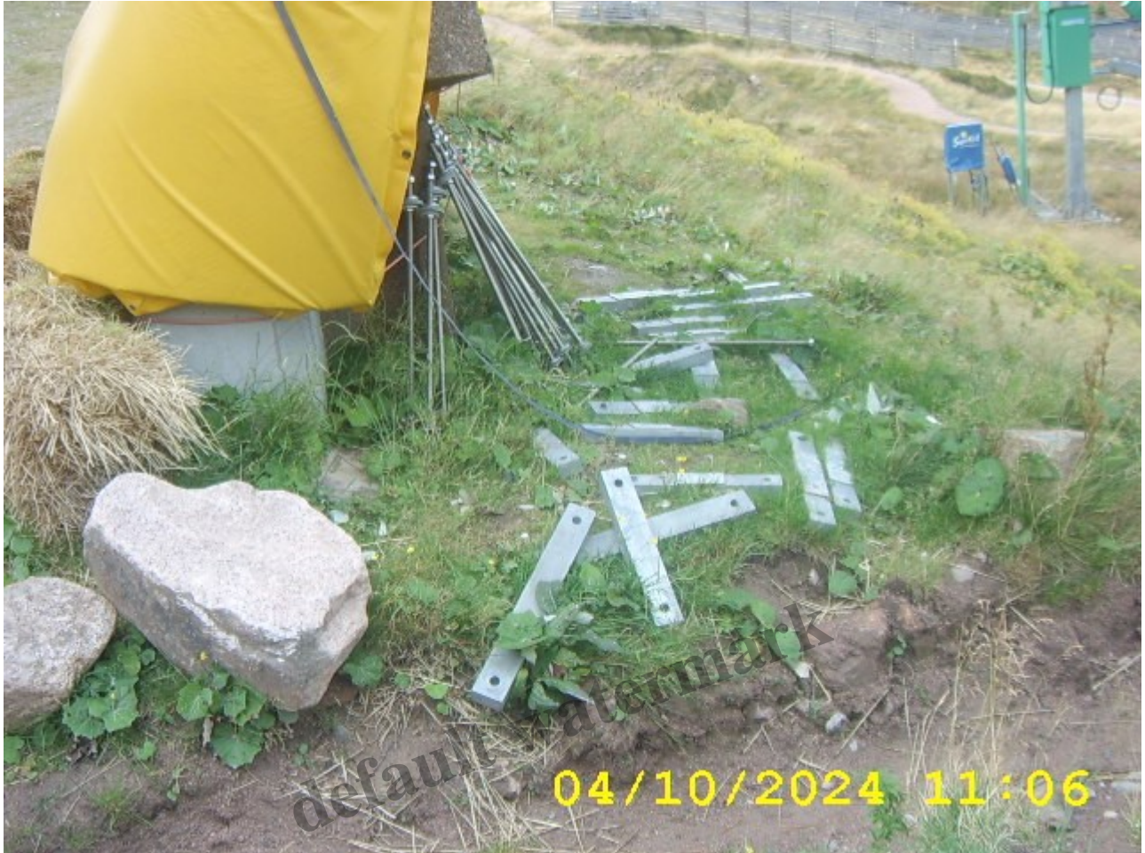
Photo. Type I brackets on the ground below Pier 47.
