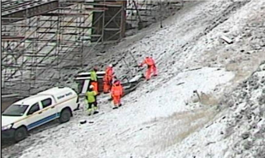
Photo 13th October – contractors appear to be working in all conditions to finish the repairs
