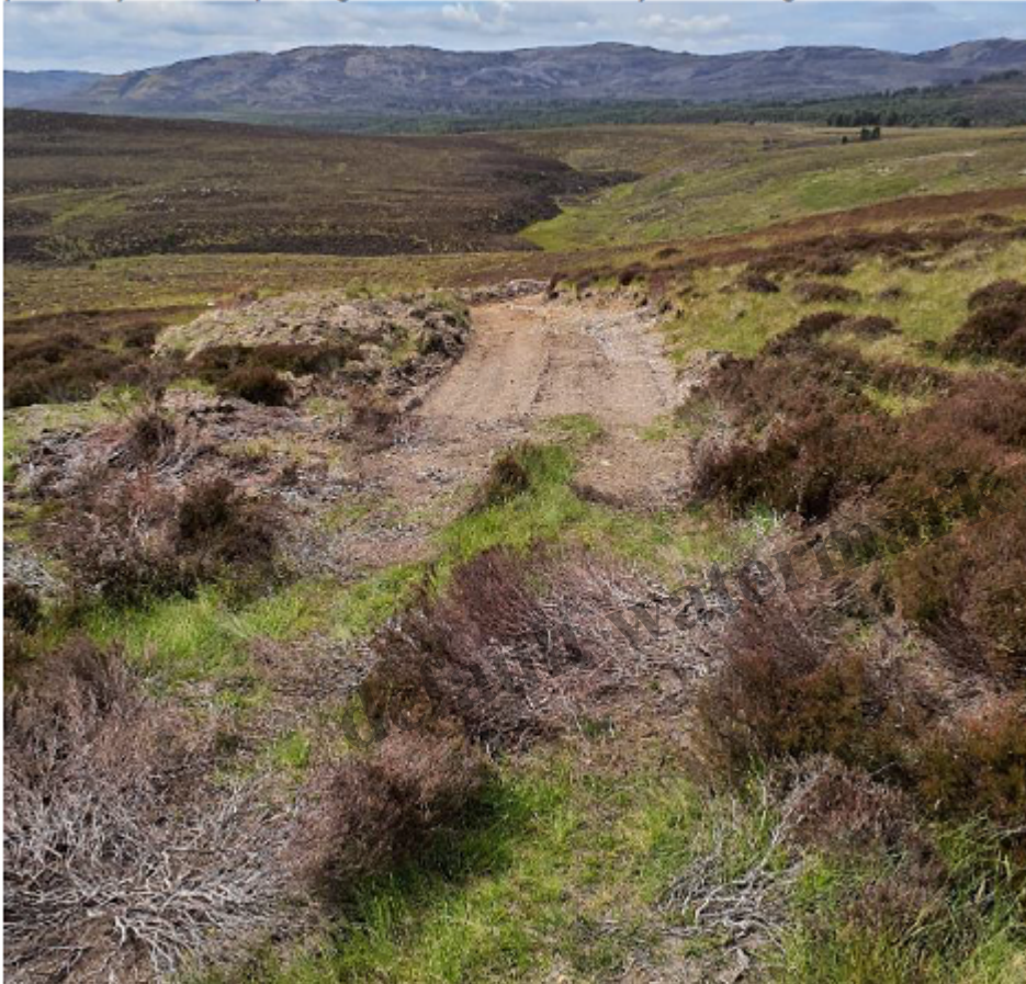
NH 9481 2942 view W Construction within close proximity to archaeological feature, potentially within no planting buffer recommended by Archaeologist.
