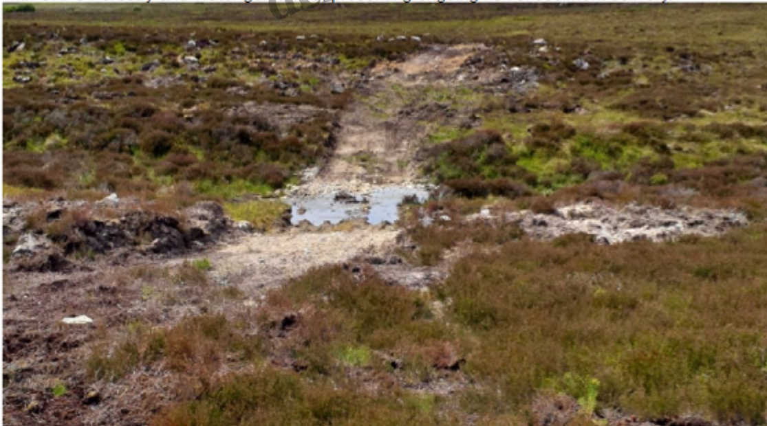
NH 9503 2819 view W Construction of new ford across Rychraggan Burn, non compliant with UKFS Forestry and Water guidelines, presenting ongoing risk of sediment delivery.
