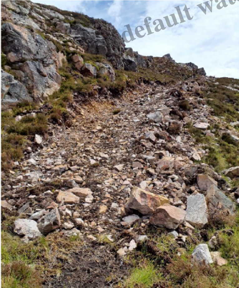
NH 9475 2962 view NE Construction on rock face below Creag an Rìgh summit
