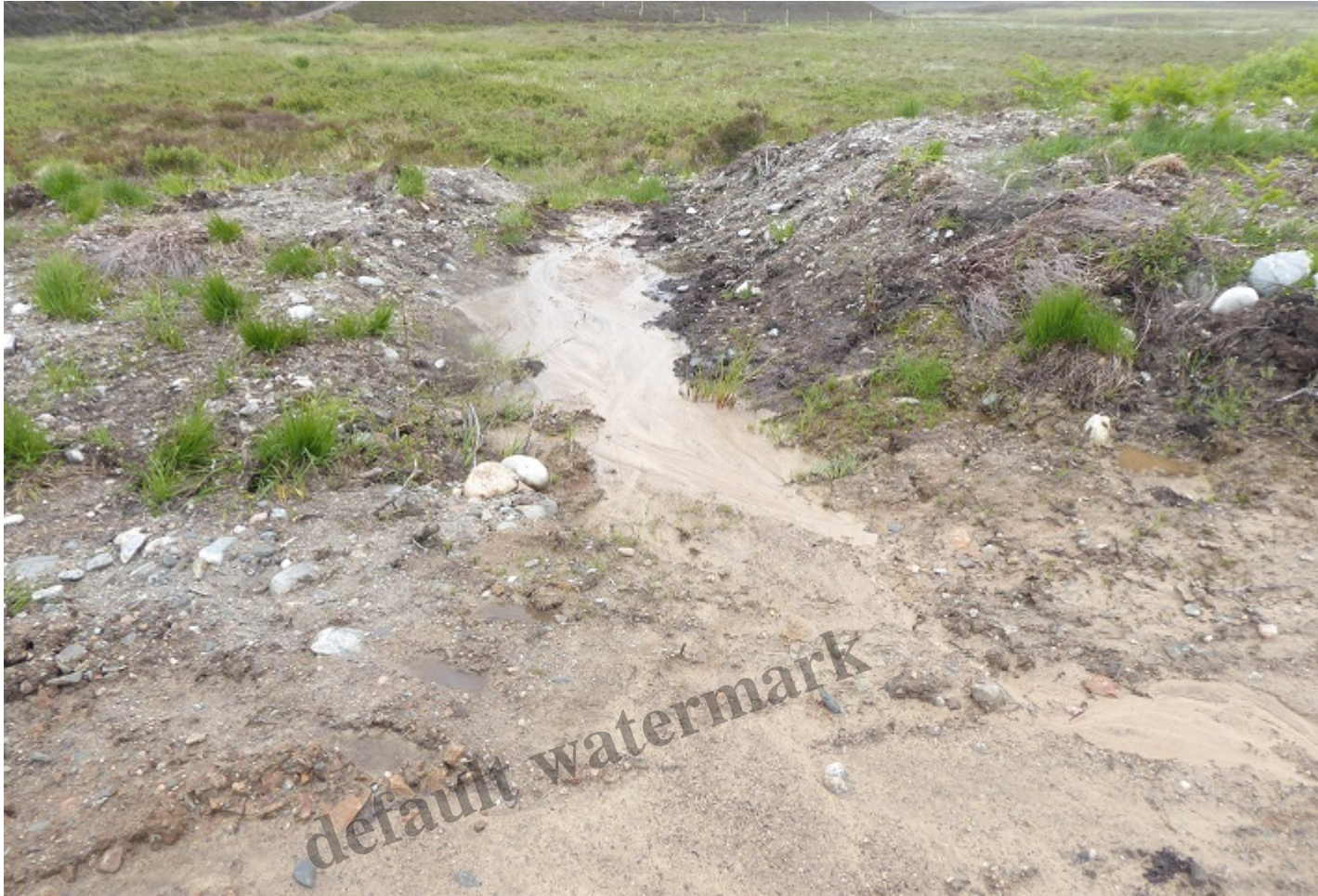
Silt washed out from the lowest drainage channel to the edge of the bog
