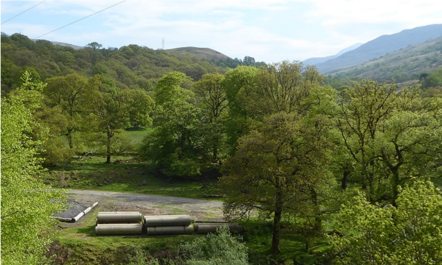
Spare pipes at the bottom of the Allt Fionn hydro track in Glen Falloch in 2018. Note the pipes are now covered with camouflage netting.
