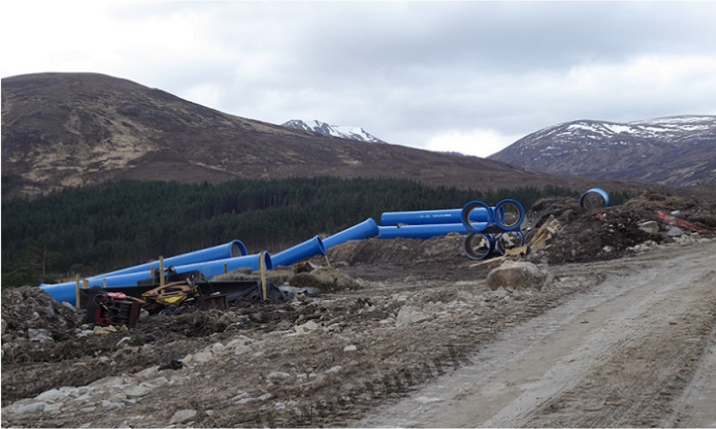
Hydro pipes during construction the construction of the Abhainn Gleann nam Fiadh hydro, Sgurr na Lapaich on left and Tom a Choinnich on right
