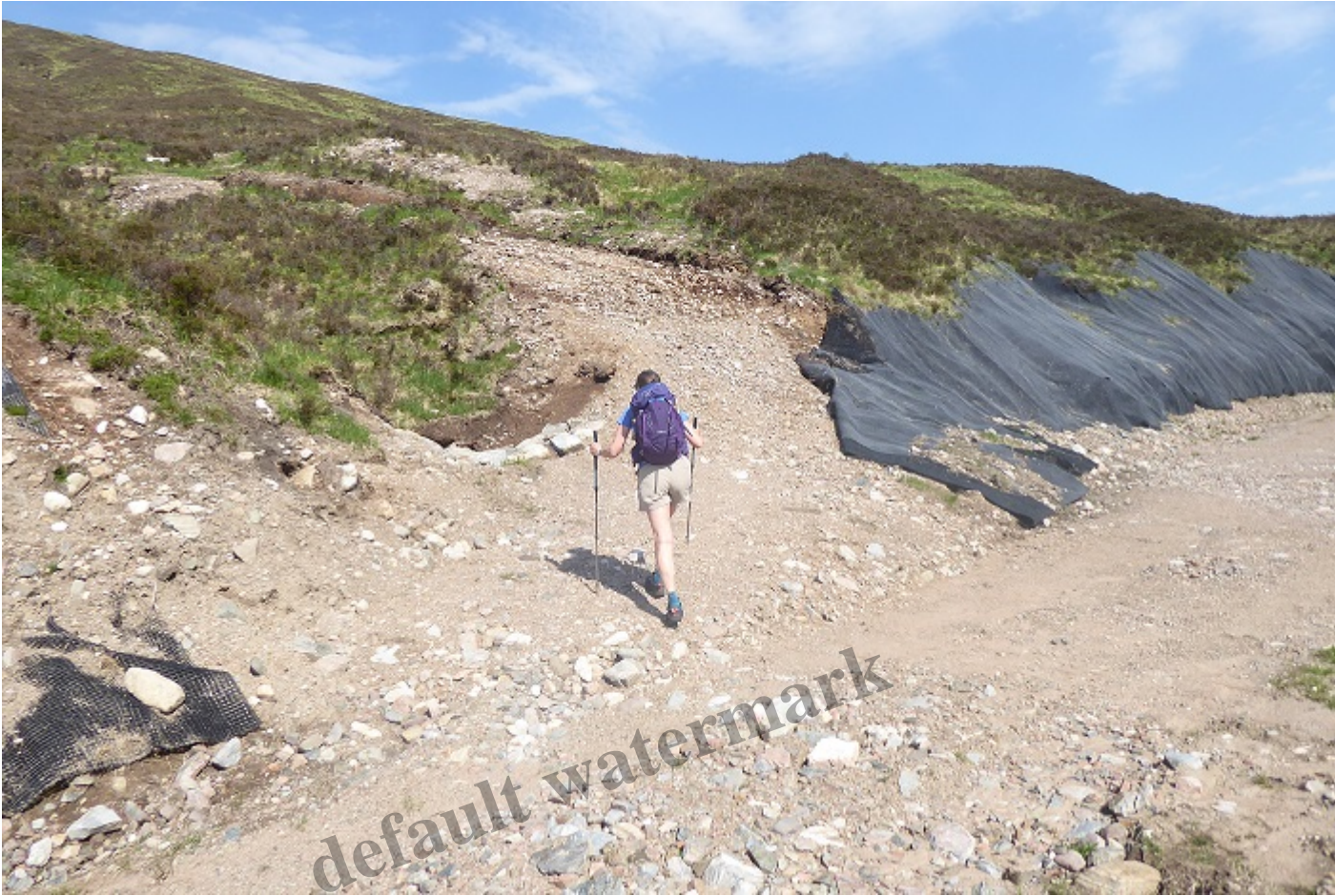
An extension of the road up onto the moorland just before the hydro intake with the plastic matting that had covered this part of the slope moved to one side
