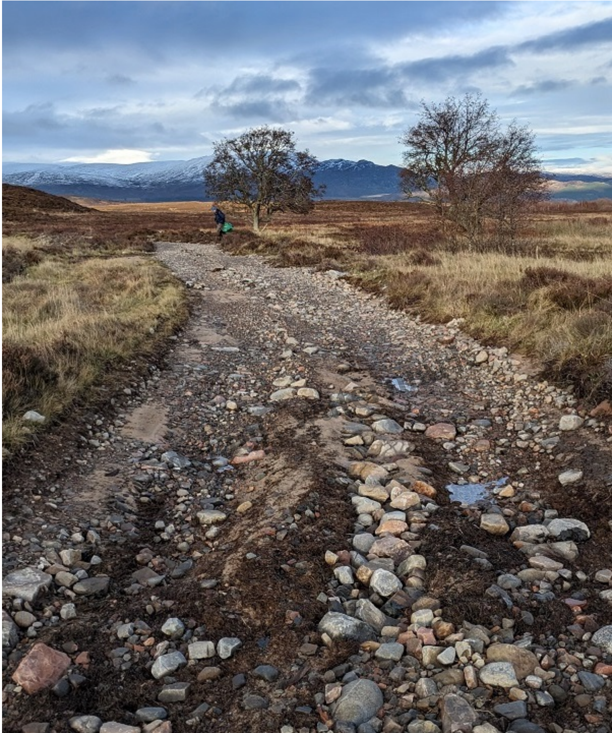
Washed out section of road by the Allt Ghuibhais
