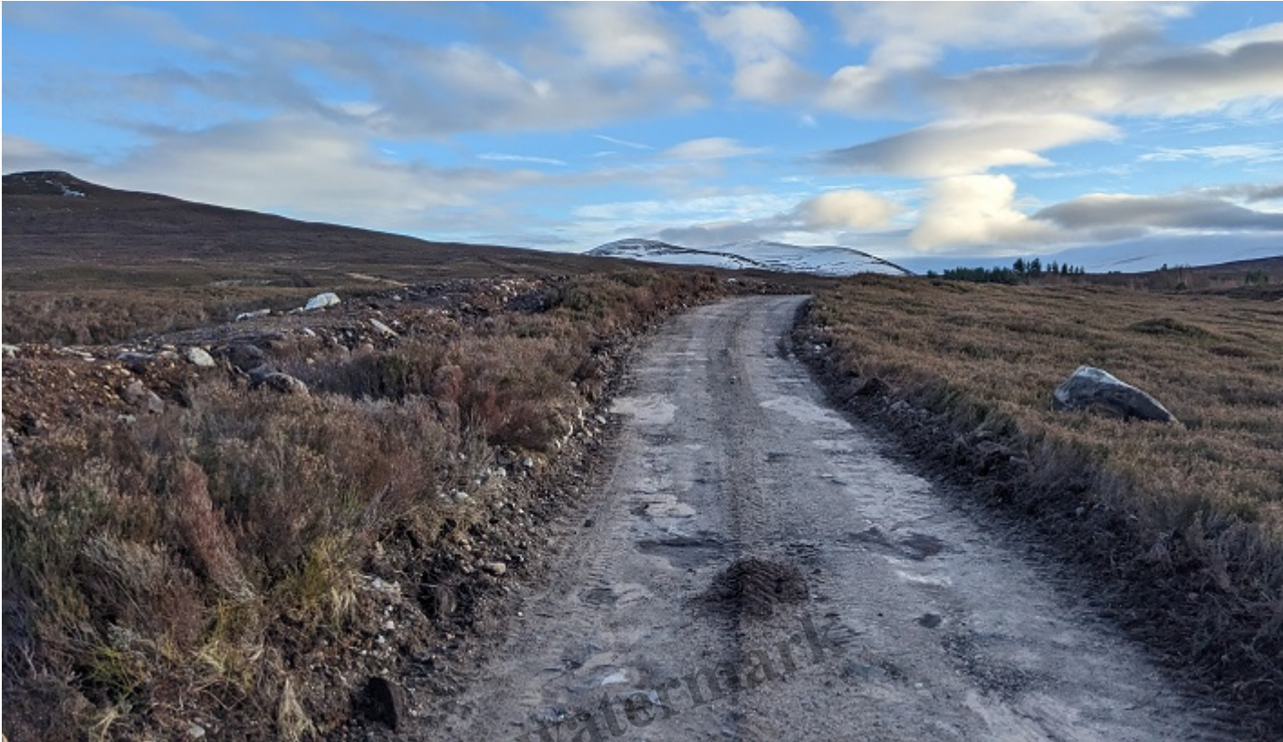
Widening and resurfacing of new road – note the new unrestored bank of soil and boulders on the left and the disappearance of the vegetated strip down the middle of the road. Photo 2nd January 2024
