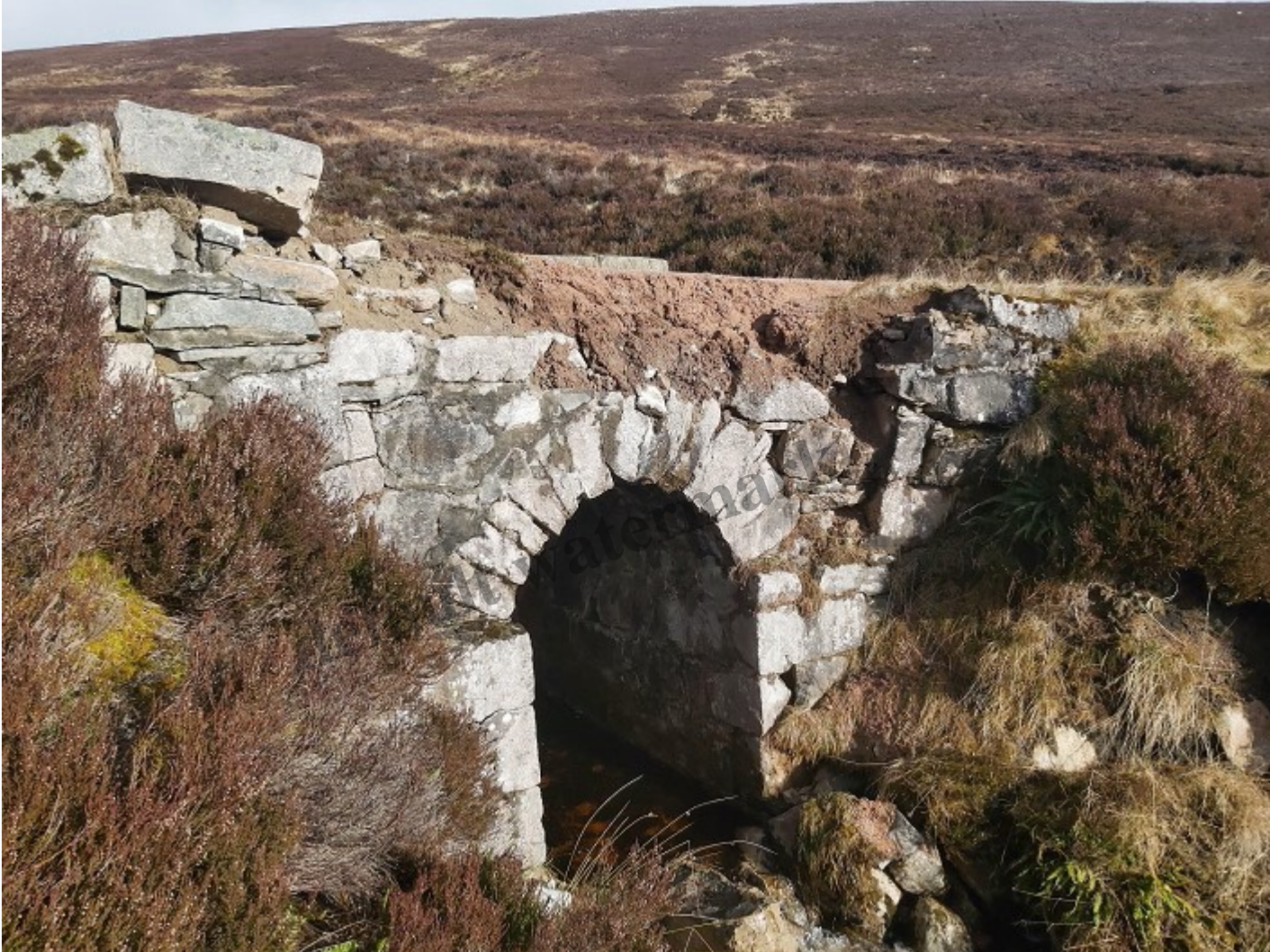
Damaged bridge on the Burma Rd. Well designed and crafted infrastructure such as this, using local materials, often enhances people's appreciation and enjoyment of the landscape. Photo credit Parkswatch reader February 2022
