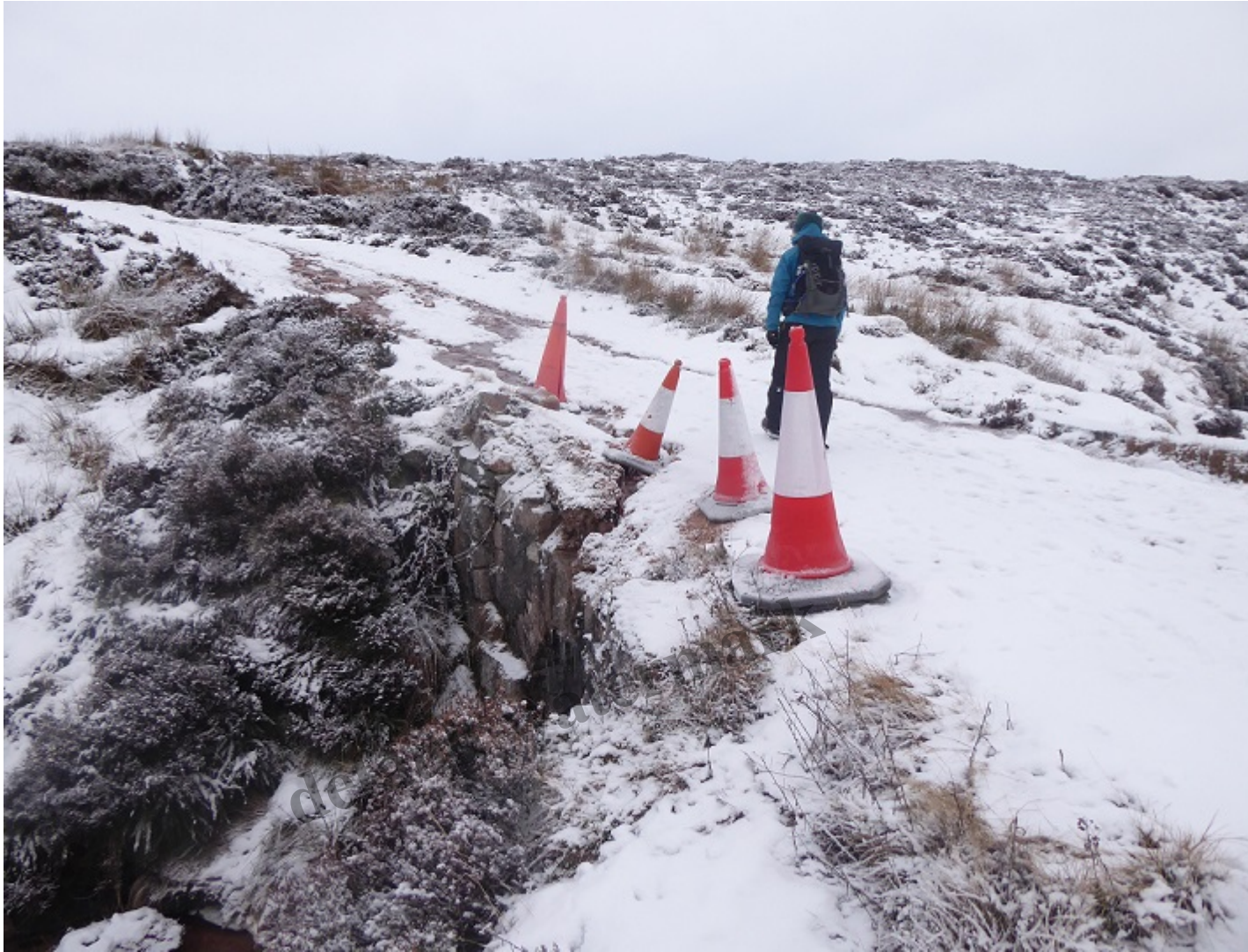
Damaged bridge December 2023
