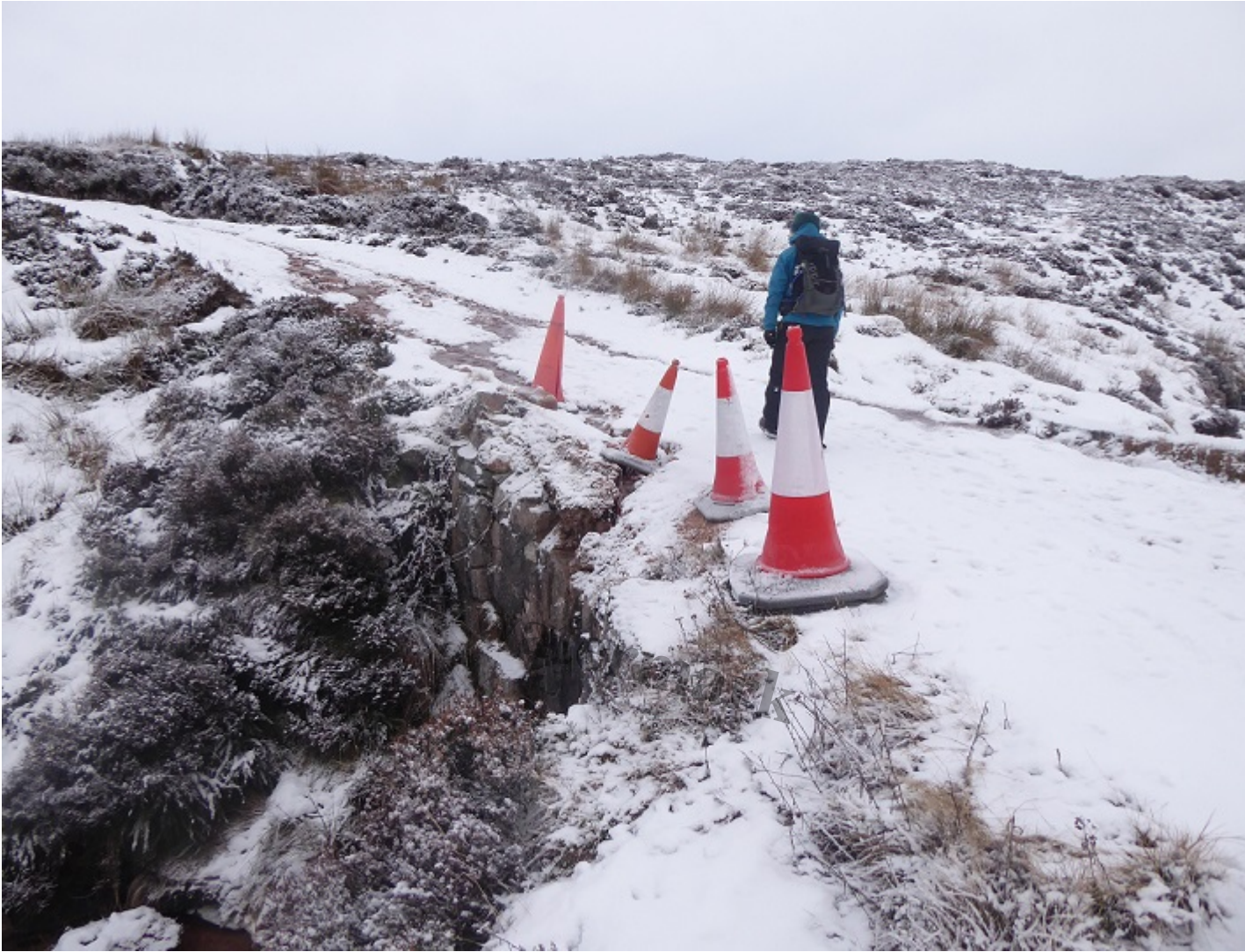
Damaged bridge December 2023
