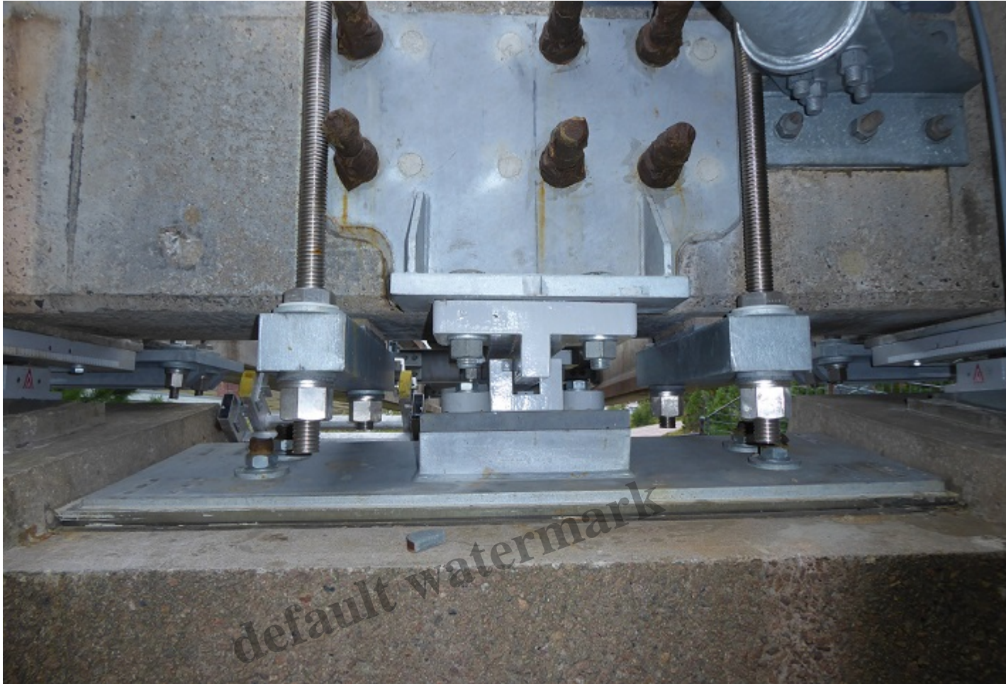
Central bearing with in situ block above and new brackets on each side
