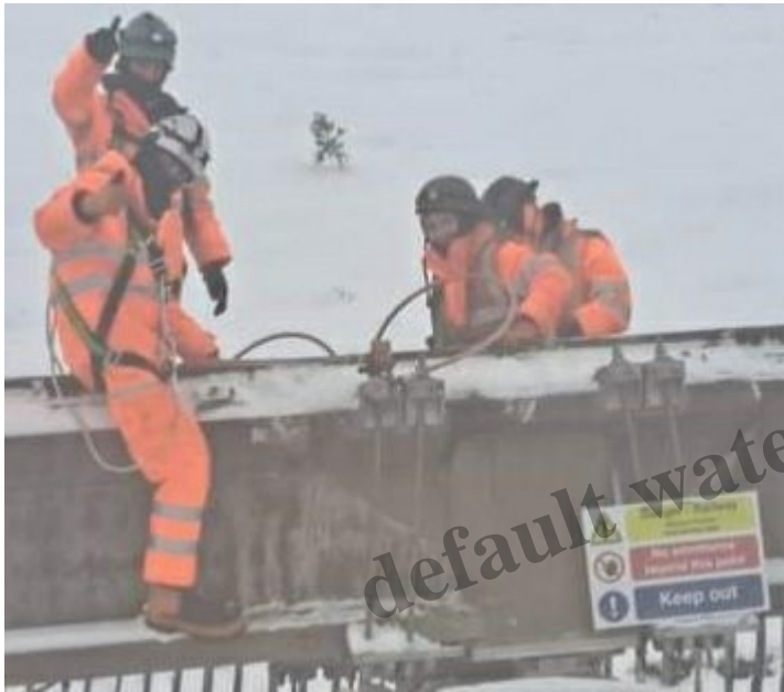
Workmen on the tracks during the w/end of 2/3 December. The metal brackets in the photo are to prevent the scarf joints breaking up.
