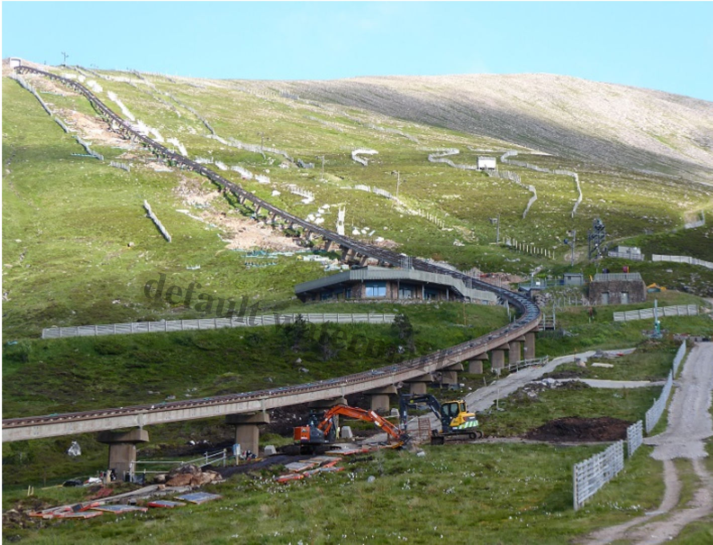
The funicular during the course of repairs July 2021. Photo credit Louise Brimelow
