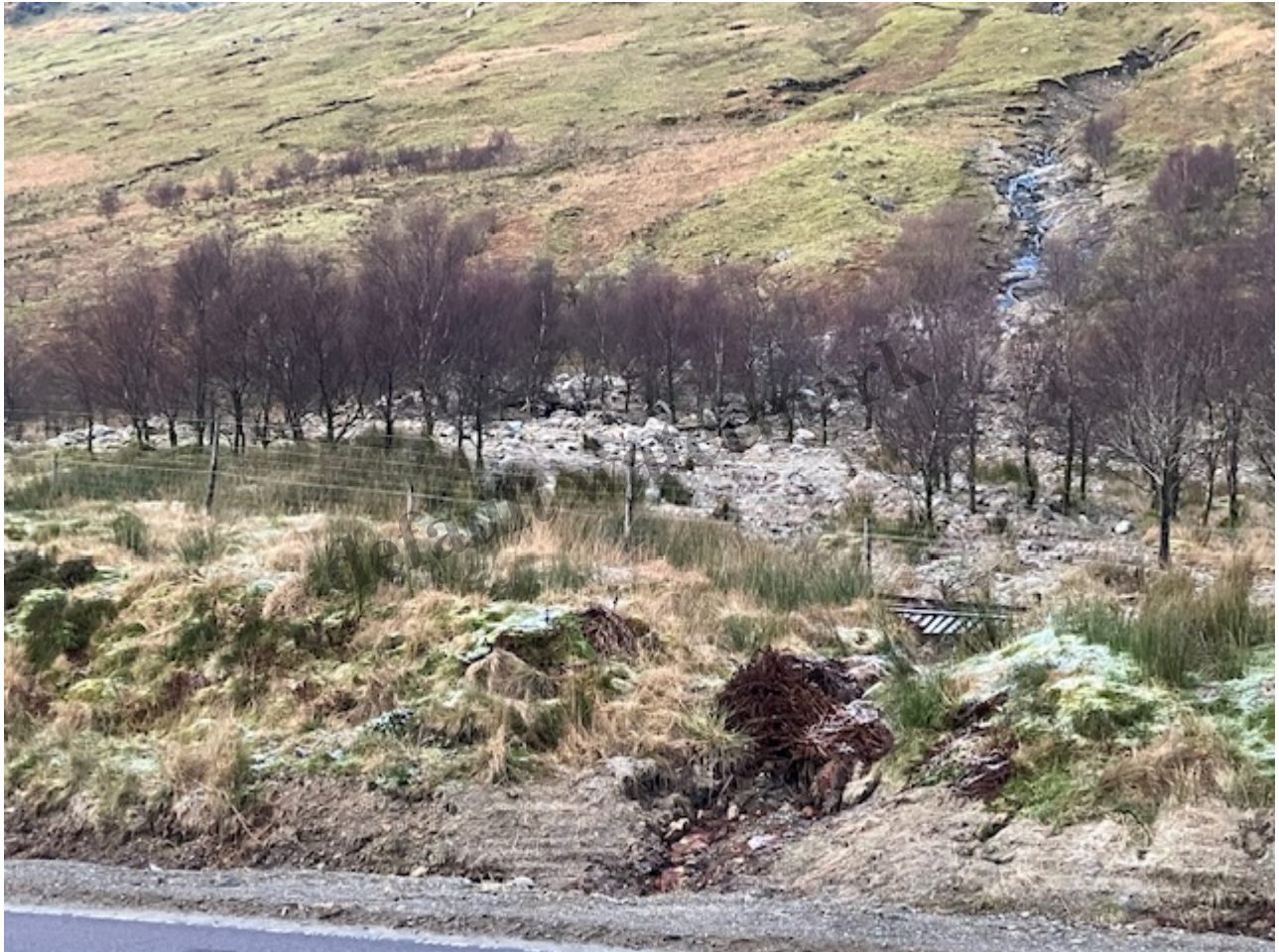
Landslip on the A83, the first below Butterbridge as you head west, viewed from the old road with the A 83 in the foreground. Photo Credit Nick Halls
