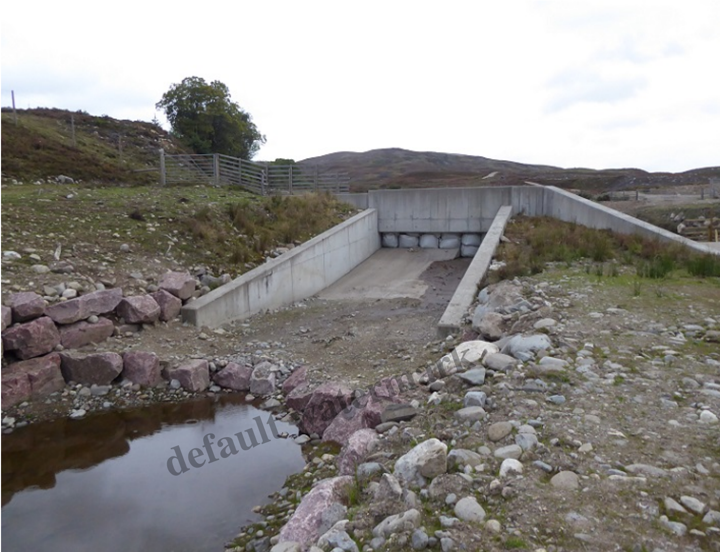
The start of the blocked overflow channel from the west September 2023
