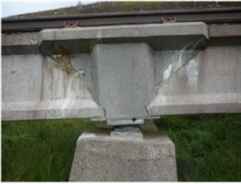
Photo [12] Pier 8, one of the poorer insitu infills. Showing joints opening between Insitu and precast plus cracking within the mass of the Insitu, both inclined and near vertical.
