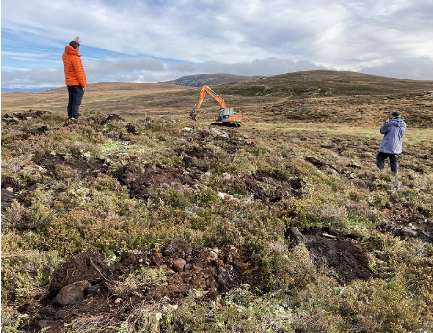
Ground preparation currently taking place on Far Ralia as part of Abrdn’s tree planting scheme. Photo which appeared in the Strathy, credit Dave Morris
