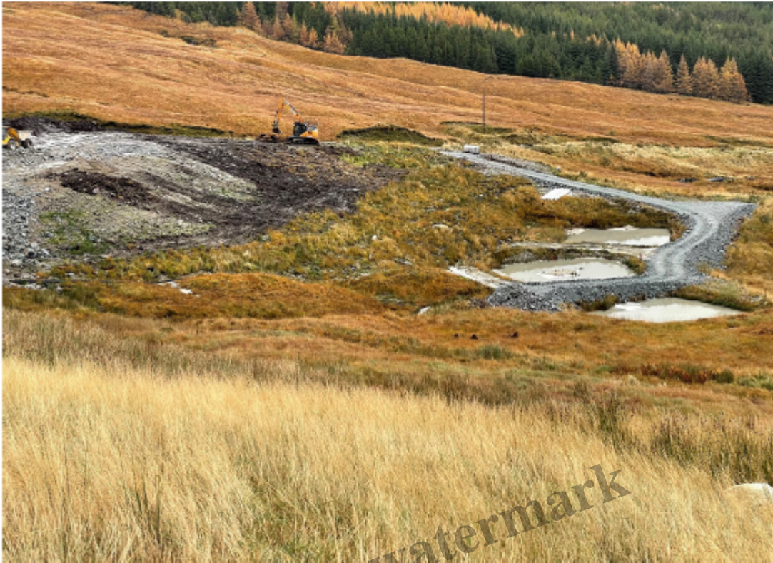
Stack 1 restoration and HEA 2 location, existing ponds to be drained prior to formation of Stack 2
