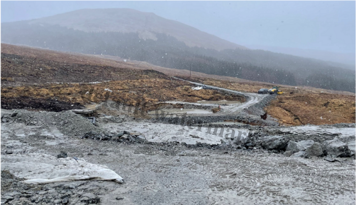
Stack 2 - Initial deposit of tailings as per KP Technical Note/ phased approach
