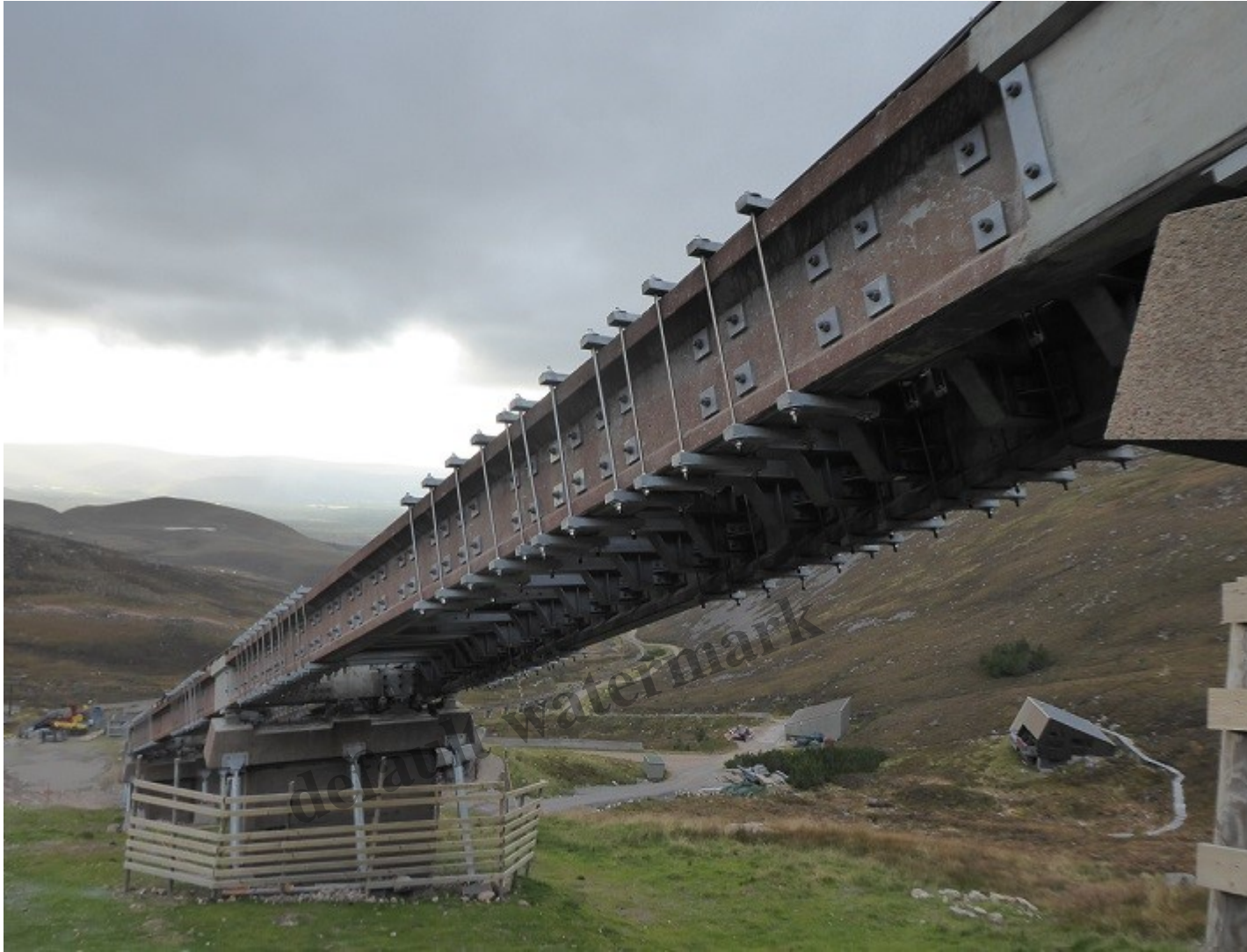
Photo showing the extensive use of metal reinforcing brackets by the mid-station
