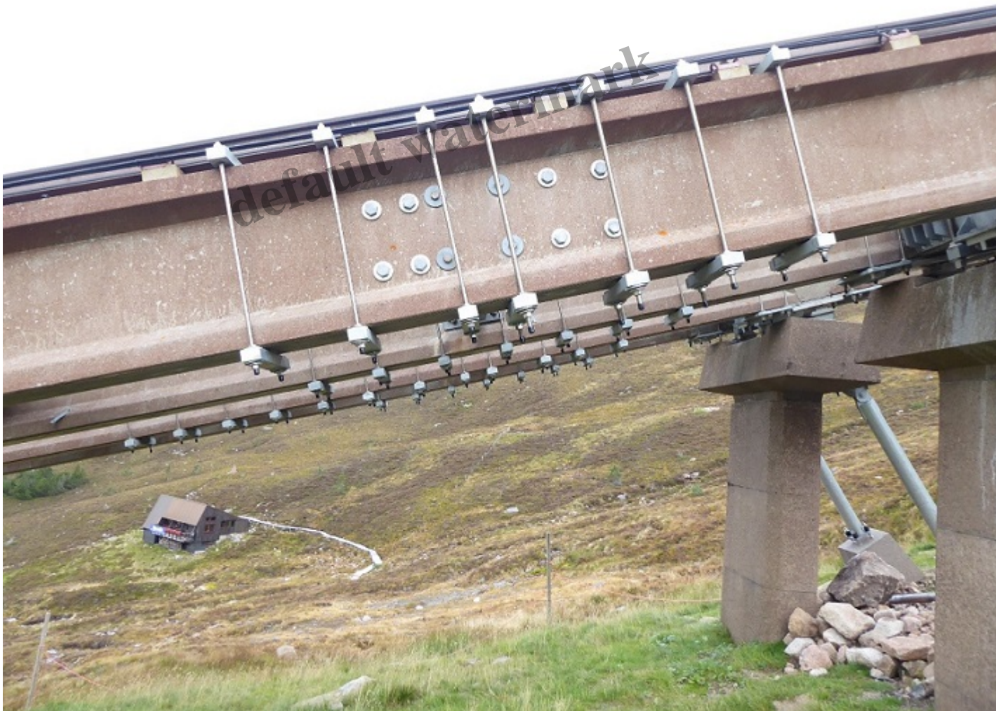
Photo showing how different additional brackets have been placed on each beam, in addition to the pairs around the scarf joints, and how the number of these brackets vary.
