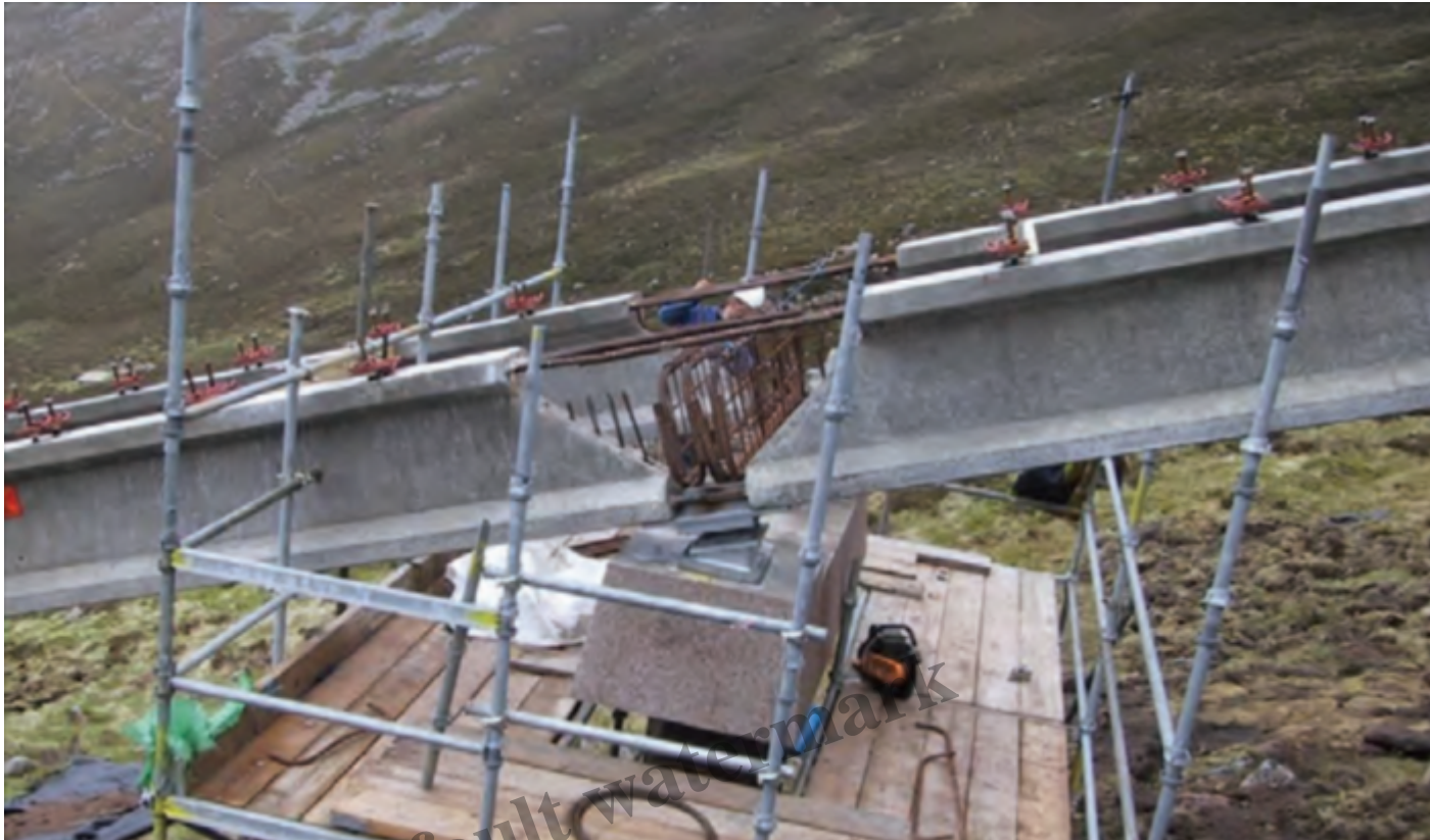
The concrete “I” beams during construction. Photo courtesy of the COWI report Dec 2018.
