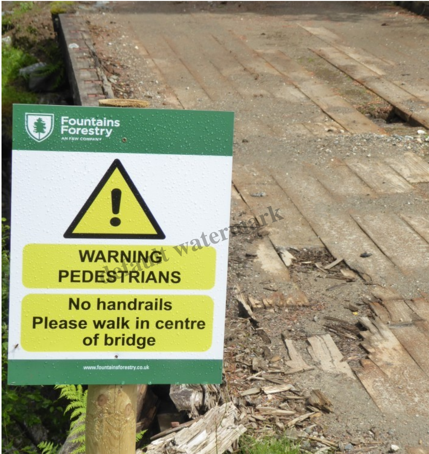
Bridge lower down the glen without safety tape. Note the hole in the centre which was large enough
