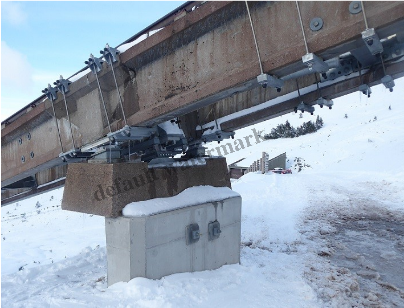
Pier below shieling with new concrete collar and metal braces on the "I" beam
