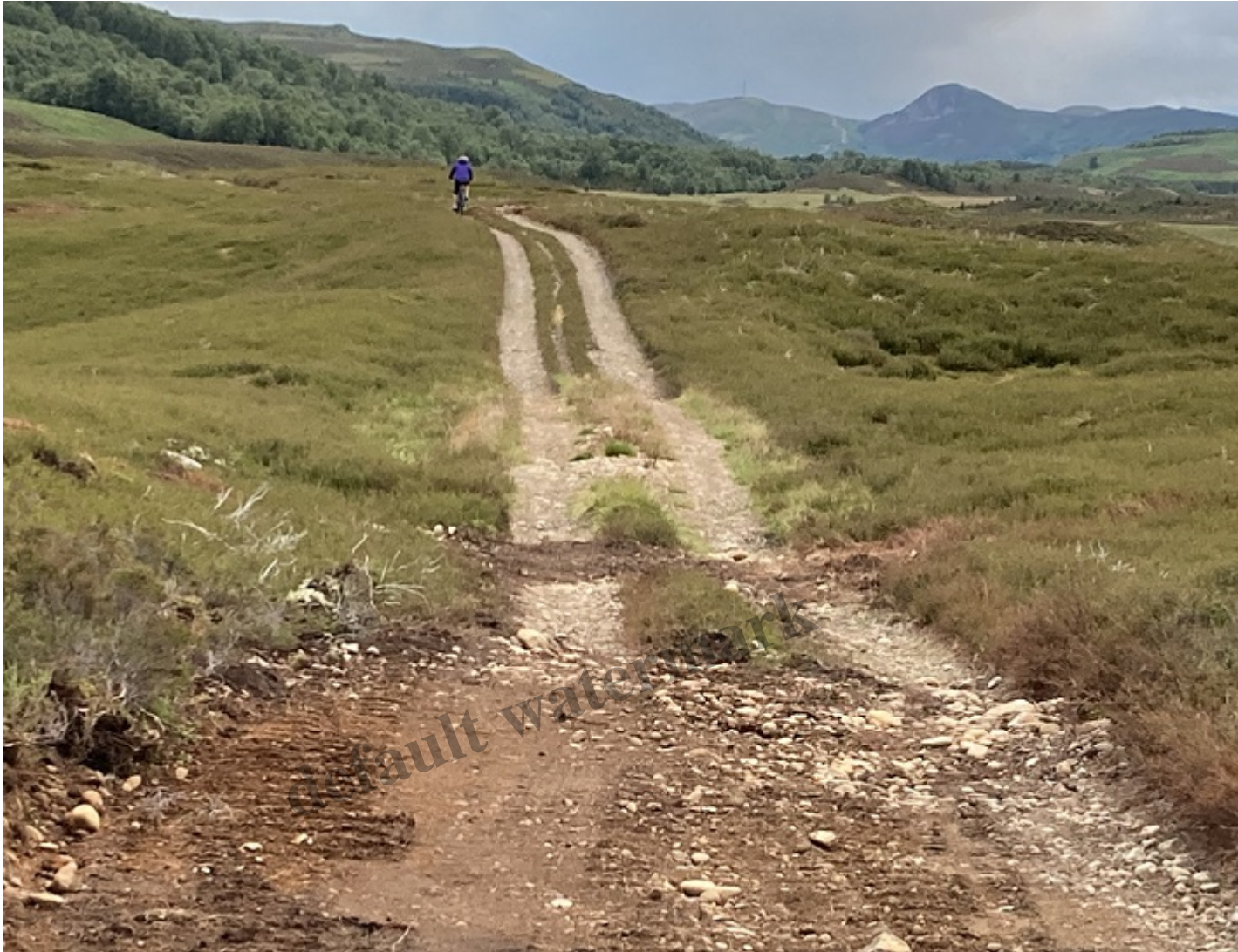
The width of the repaired road is clearly significantly greater than the existing road
