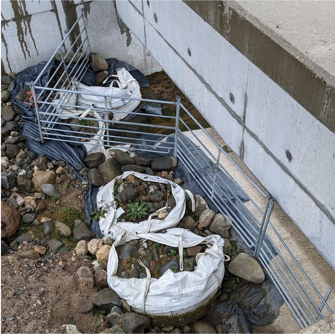
The blocked up intake 2022
