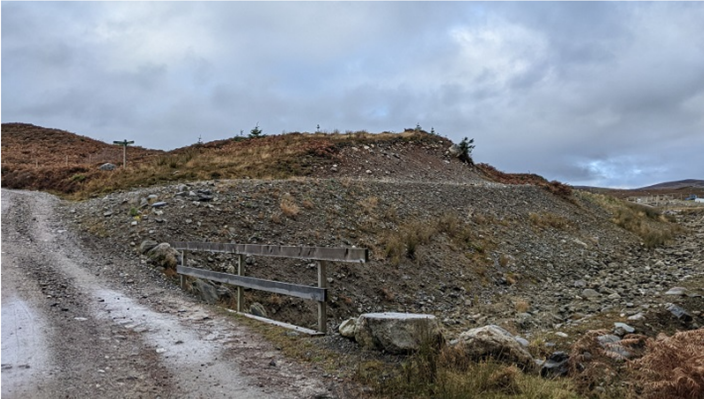
Unrestored bank and track cutting just below the intake to the channel. November 2022.
