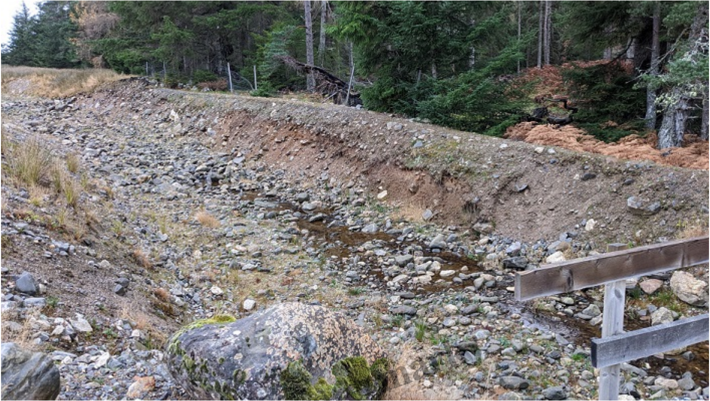
The upper part of the diversion channel with a heavily eroded section of the channel containment bund on the right. Photo Nov 2022.
