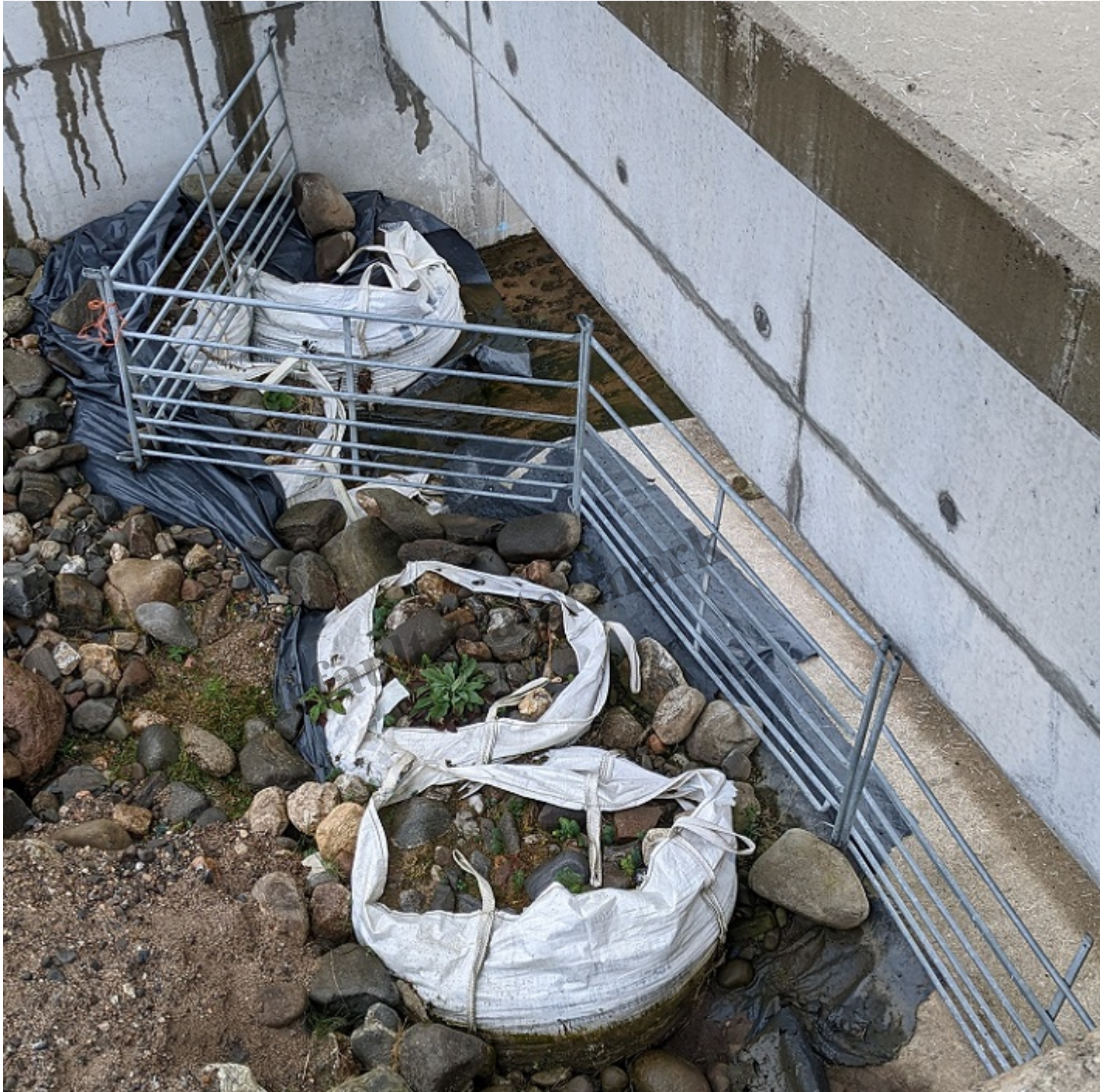
The blocked off intake by the River Gynack November 2022.
