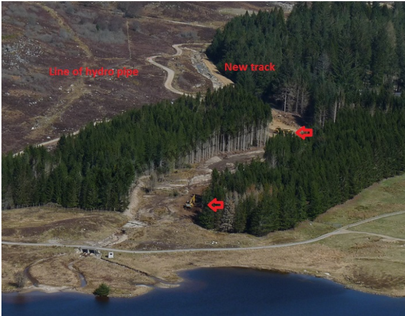
View of Gynack flood alleviation channel from Creag Bheag, April 2023, showing JCB, Truck and new track alongside it. Loch Gynack in foreground. Photo credit parkswatch reader.
