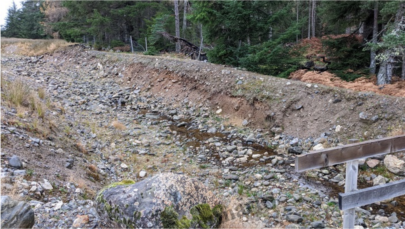
The upper part of the diversion channel with a heavily eroded section of the channel containment bund on the right. Photo Nov 2022.
