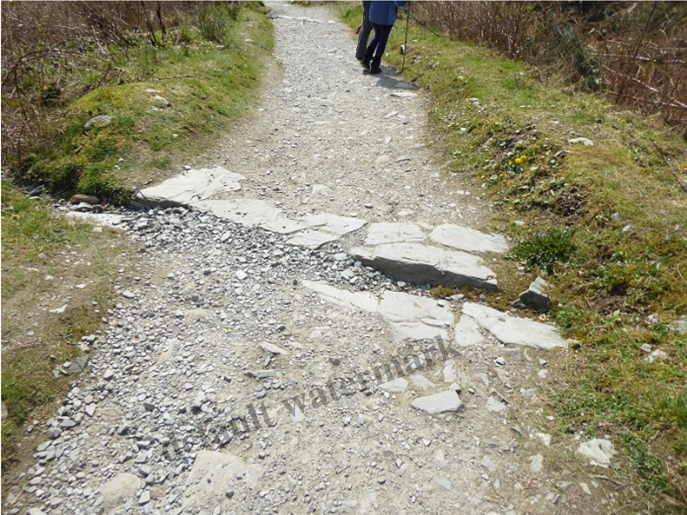
Cross drain clogged up with eroded material
