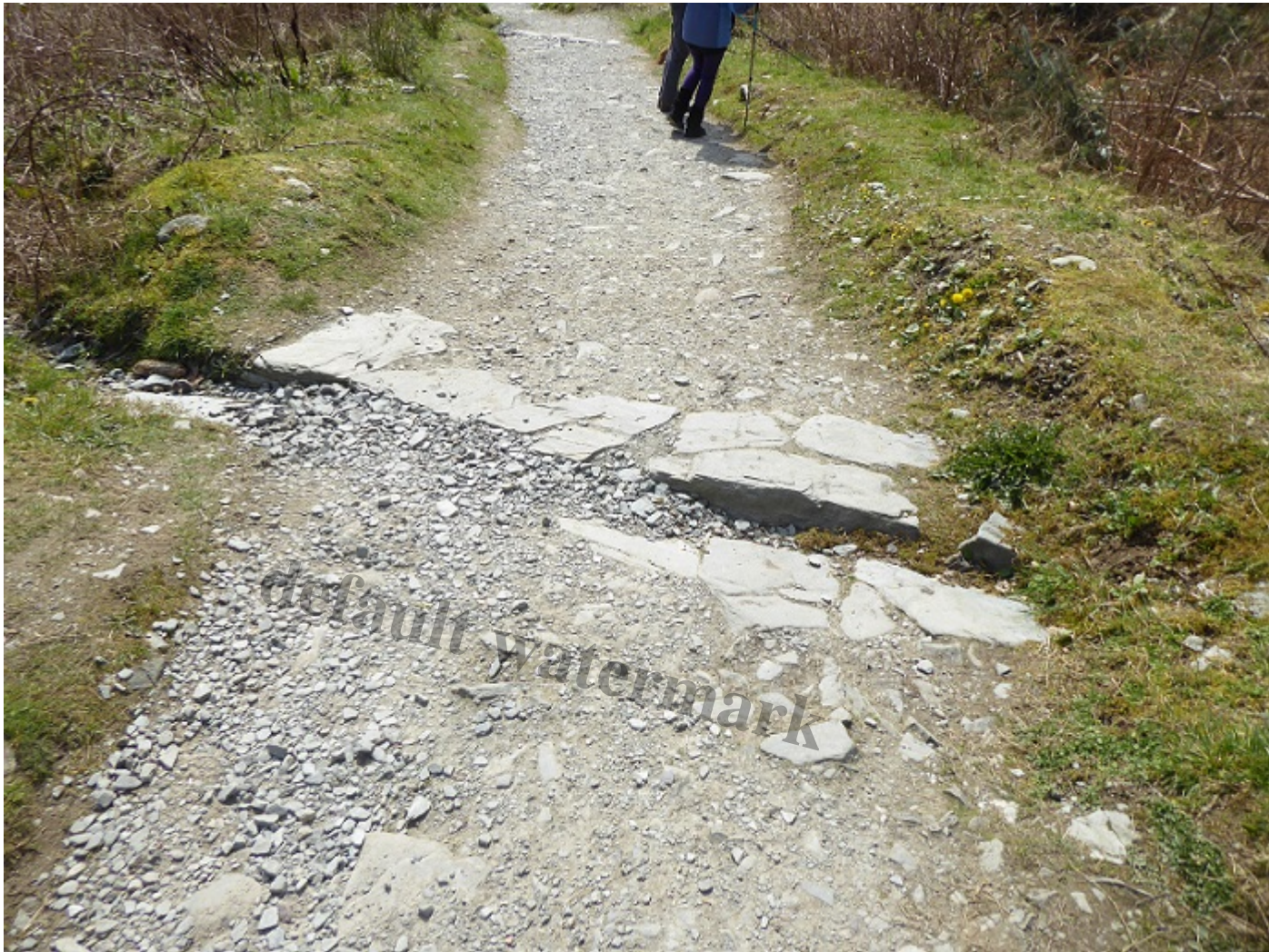
Cross drain clogged up with eroded material
