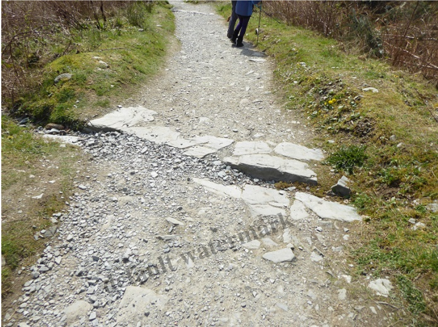
Cross drain clogged up with eroded material
