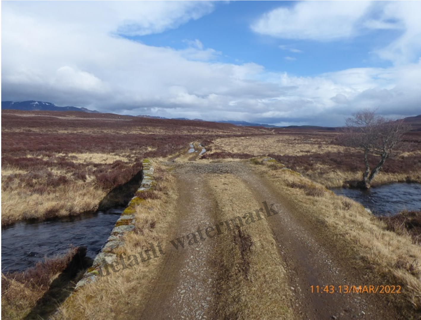
The track and former military road as it crosses the Wade bridge
