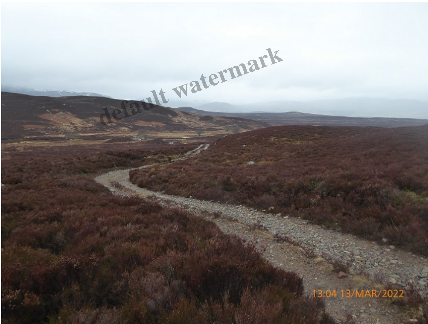
View back along the first part of the upper section of track – it winds over the shoulder of the hill in the middle ground. What needs repaired here?
