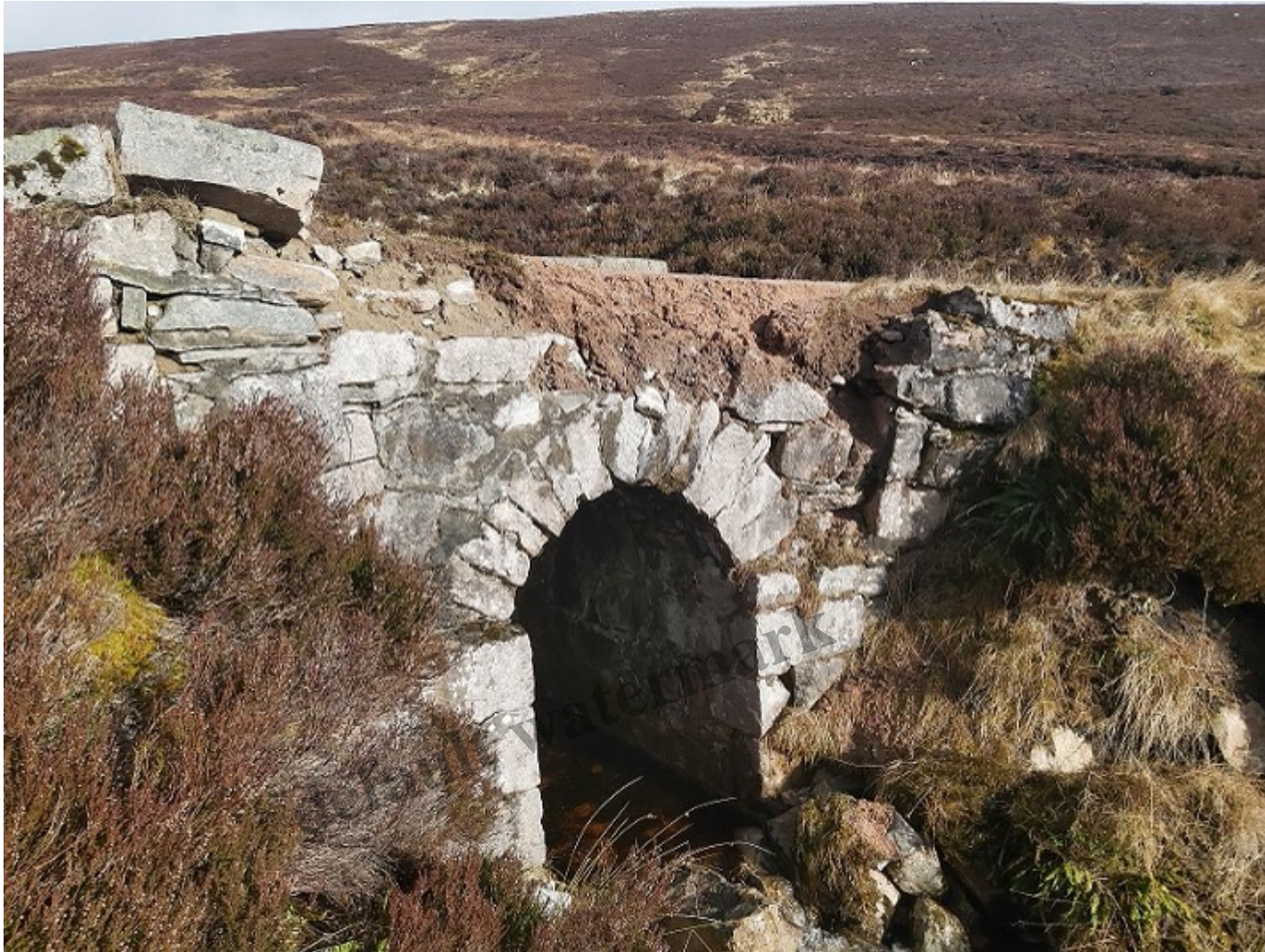
The crushed parapet of the bridge. Photo credit parkswatch reader.
