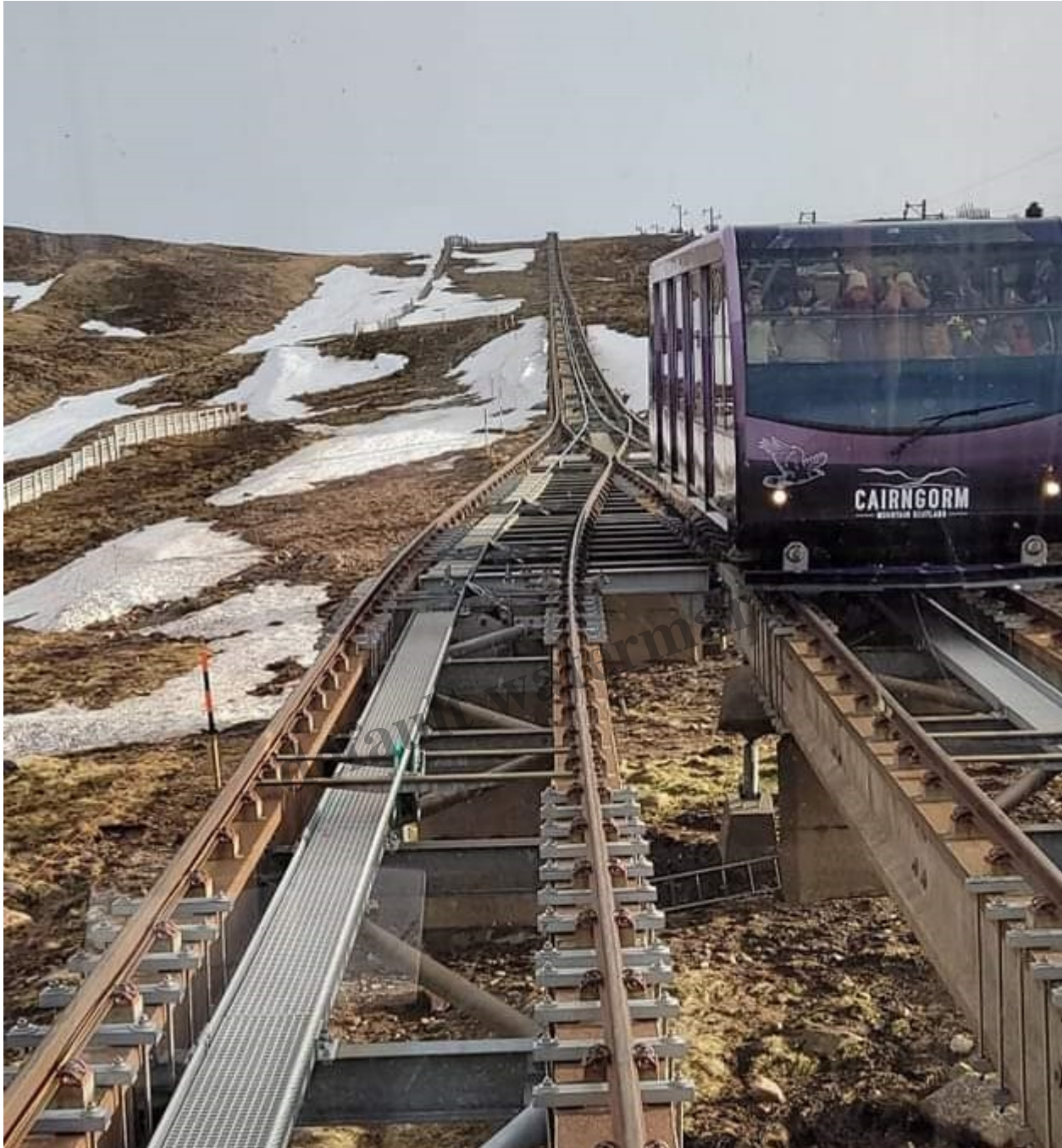
The new walkway and lots of metal brackets. Incidentally, note the state of the ground below! Photo from FB
