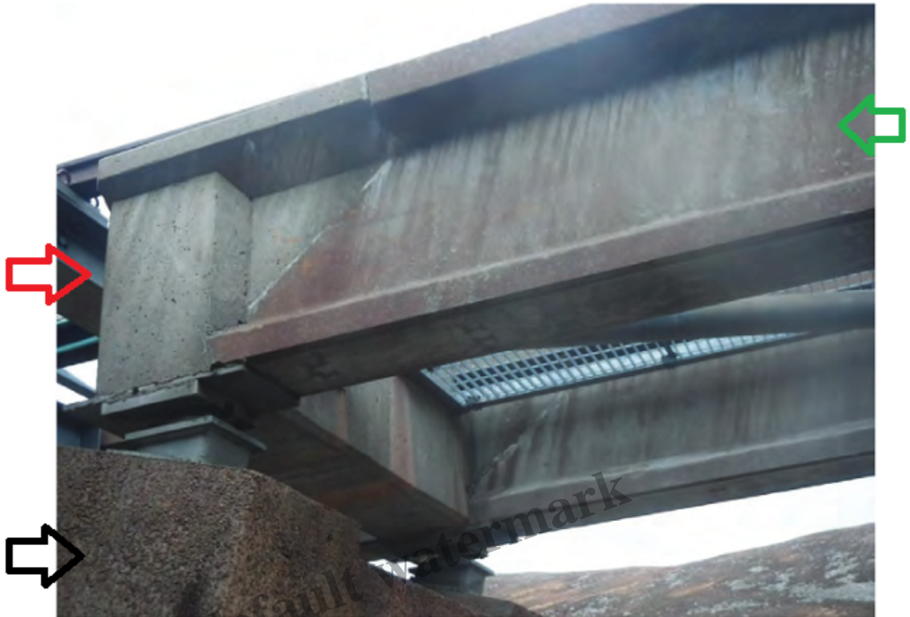
Plate 24 - General view of surface markings to Pier 53 Right Beam, left support up.
