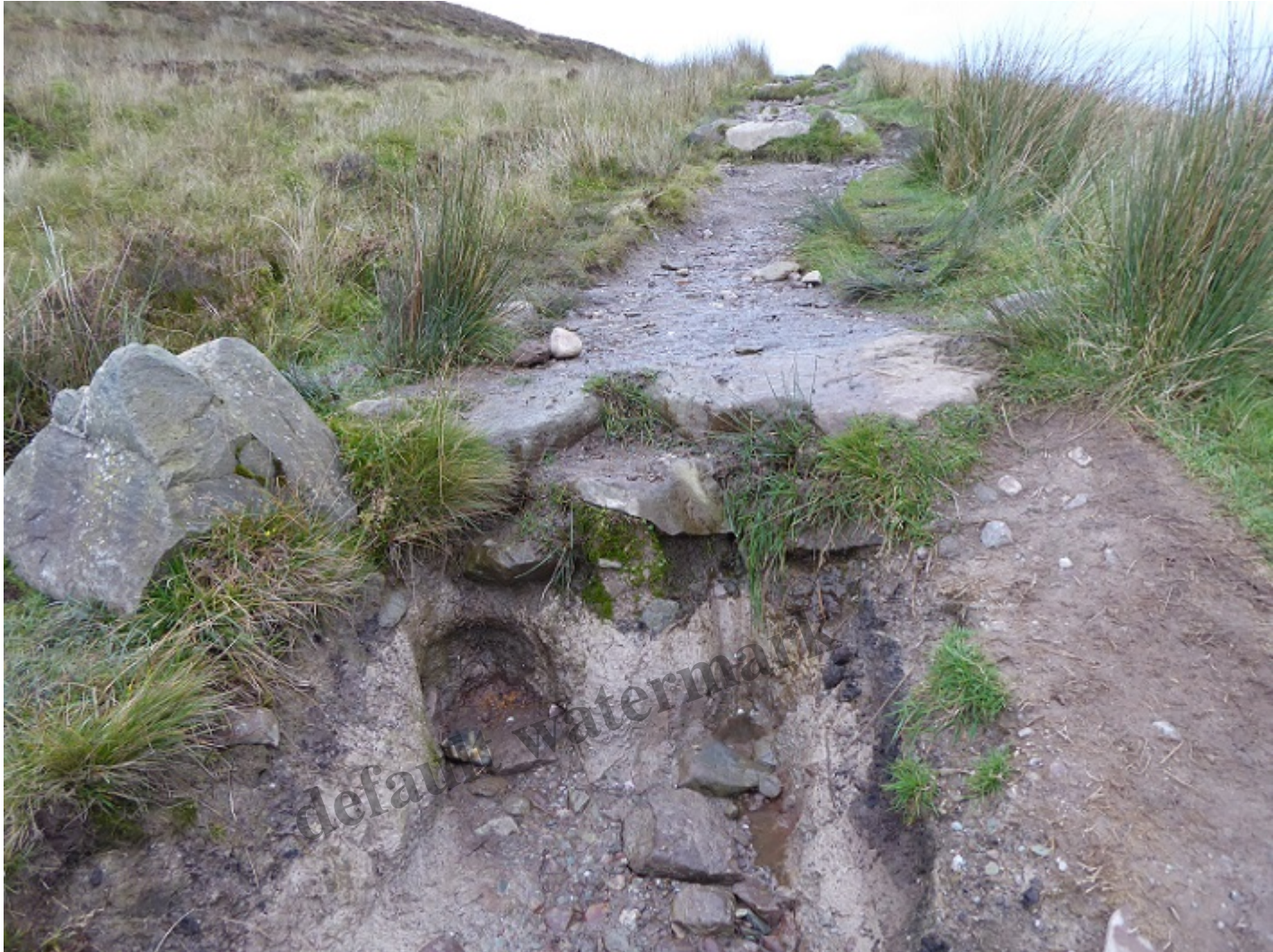
Filling up the hole with aggregate will not solve the problem, this needs stone pitch steps plus the creation of effective waterbars. Photo October 2020
