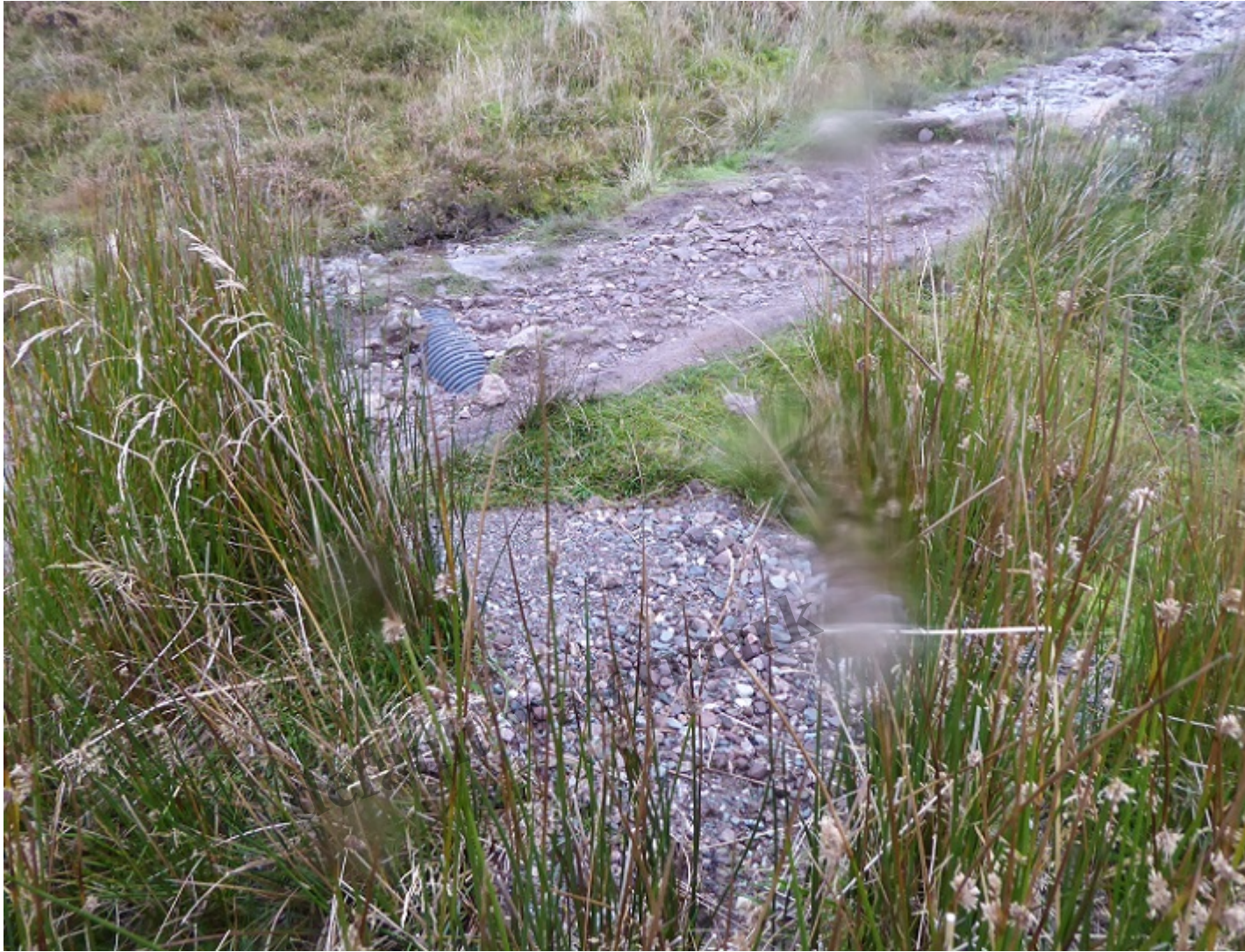
Evidence of surface wash out. Some of the finer material is likely to have found its ways down into the Burn of Mar and the River Endrick Special Area of Conservation
