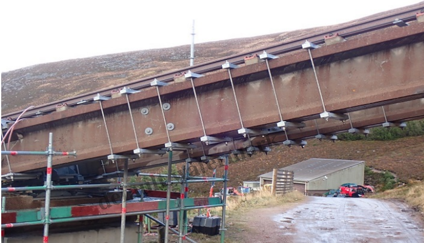
Photo 1. Steel braces reinforcing the “I” beam: there are seven visible on the near beam, eight on the beam behind. What are they all for? Photo credit Parkswatch reader.
