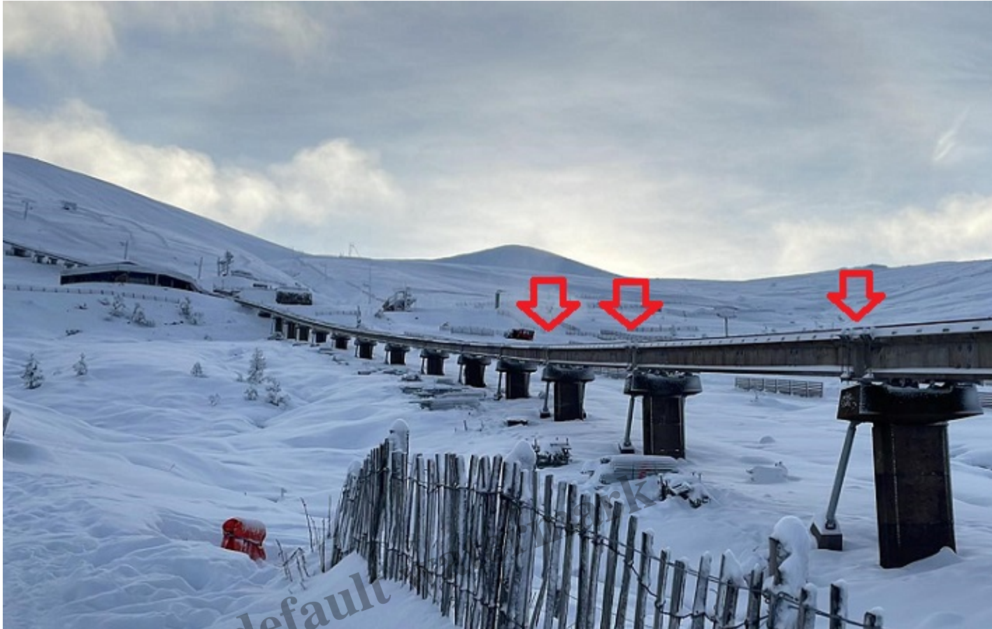
Photo (4) Red Arrows point to reinforcing by insitu blocks. Photo credit parkswatch reader.
