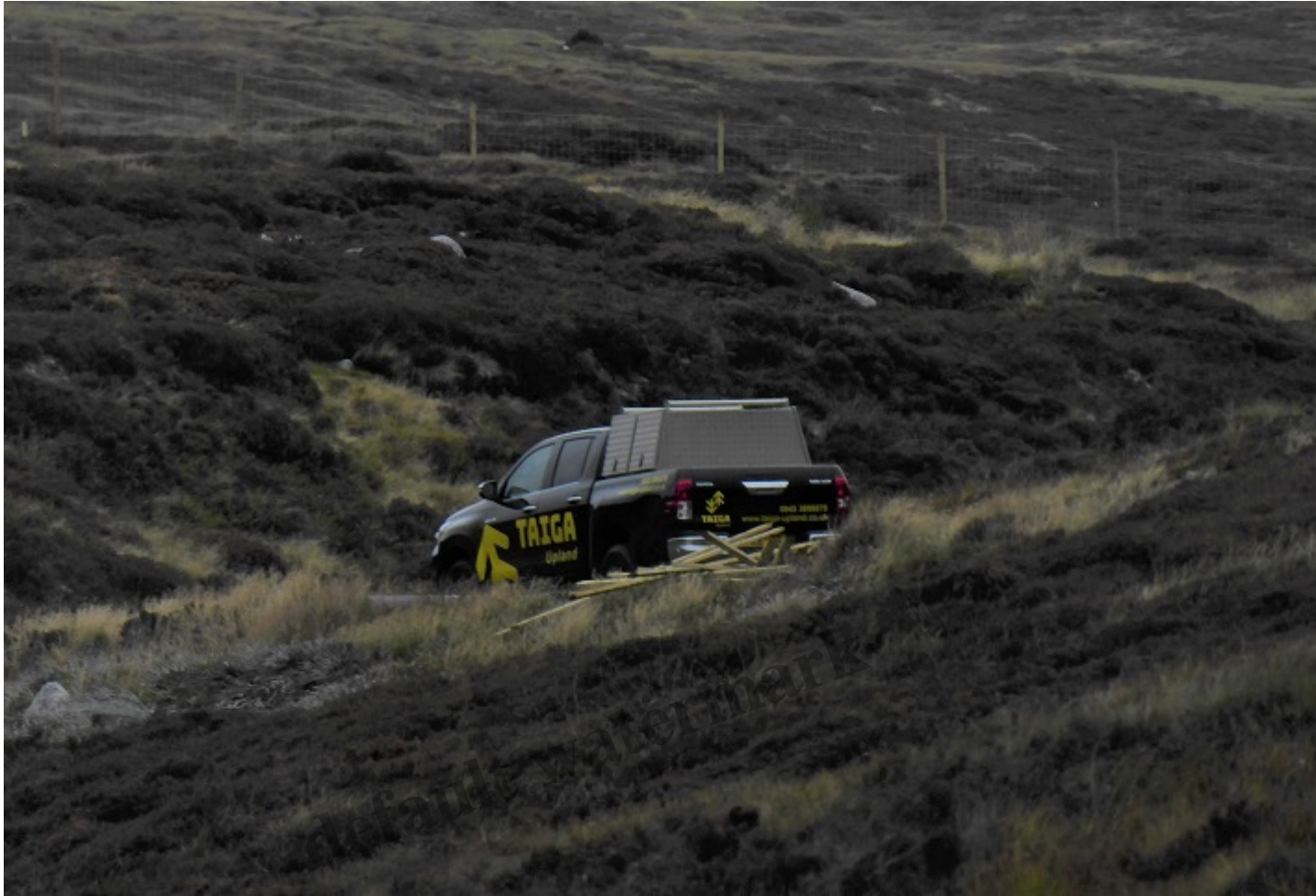
The erection of new deer fences on BrewDog's estate at Kinrara. Photo September 2022.
