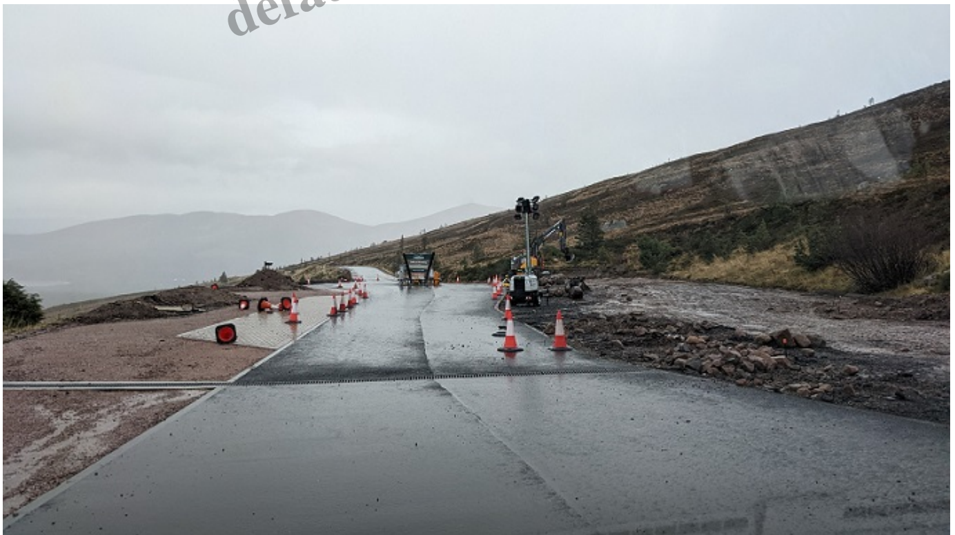
Looking towards the exit to the car park, with new hardstanding on right.
