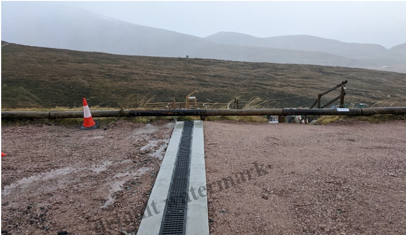
Unfinished work with the drain line protruding above the surrounding ground. Note how water is already eroding the surface on the left.
