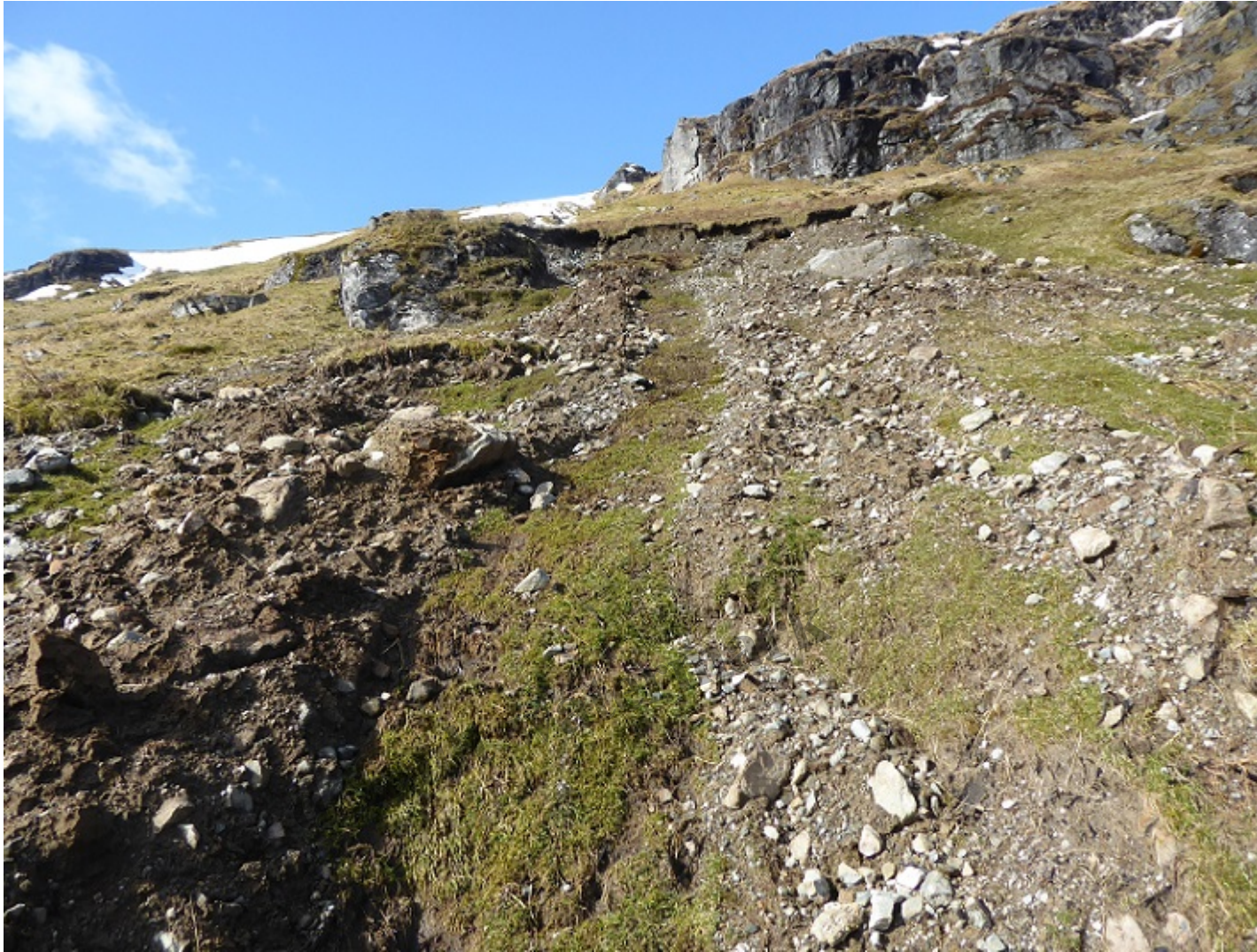
Landslip on south slope of Beinn a Chroin. Note how the volume of water has washed clean a strip down the centre of the landslip. March 2020.
