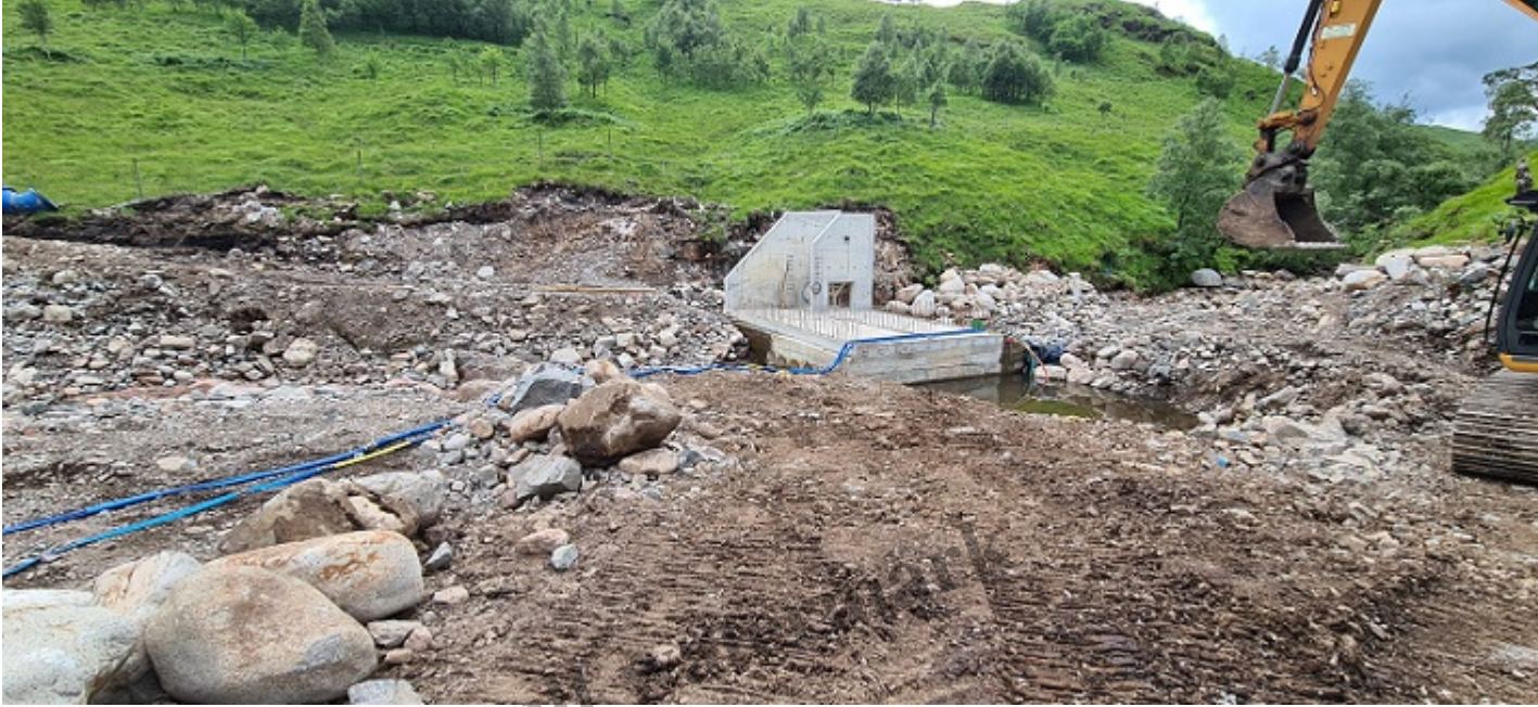
The main/primary intake
