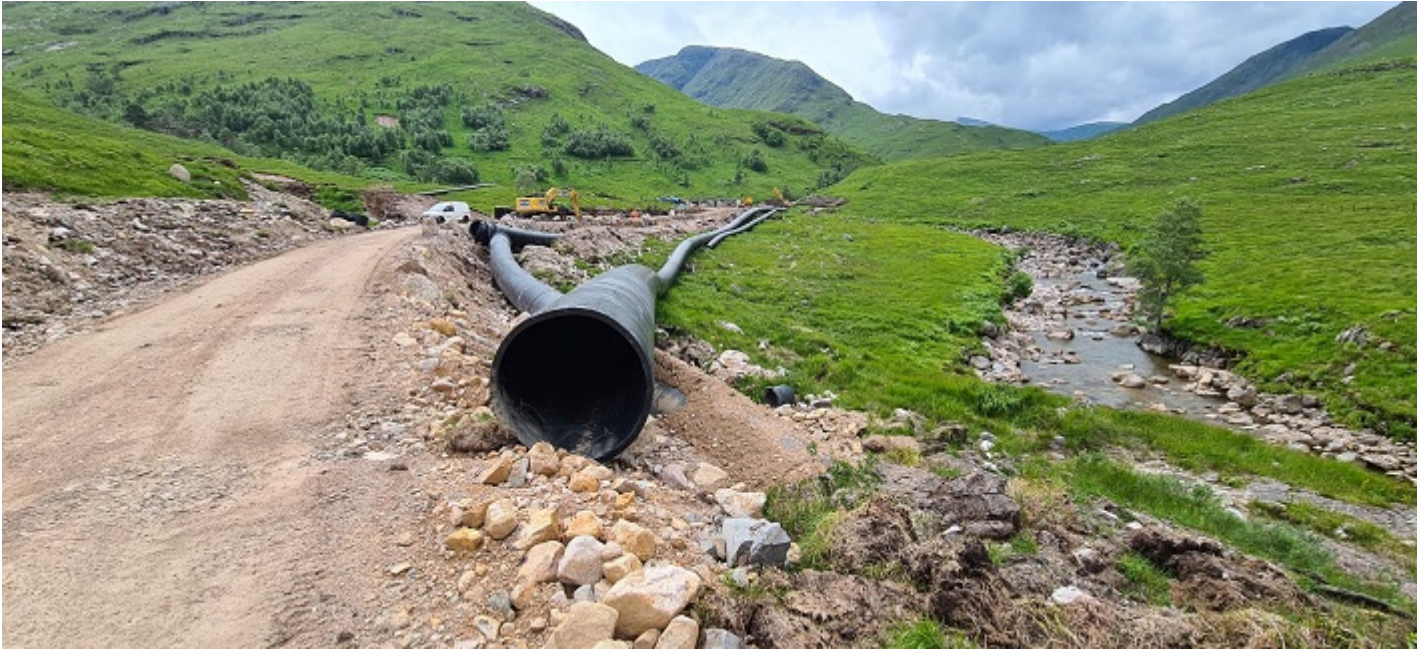
View along the construction corridor up to the intakes with excavated peat on right
