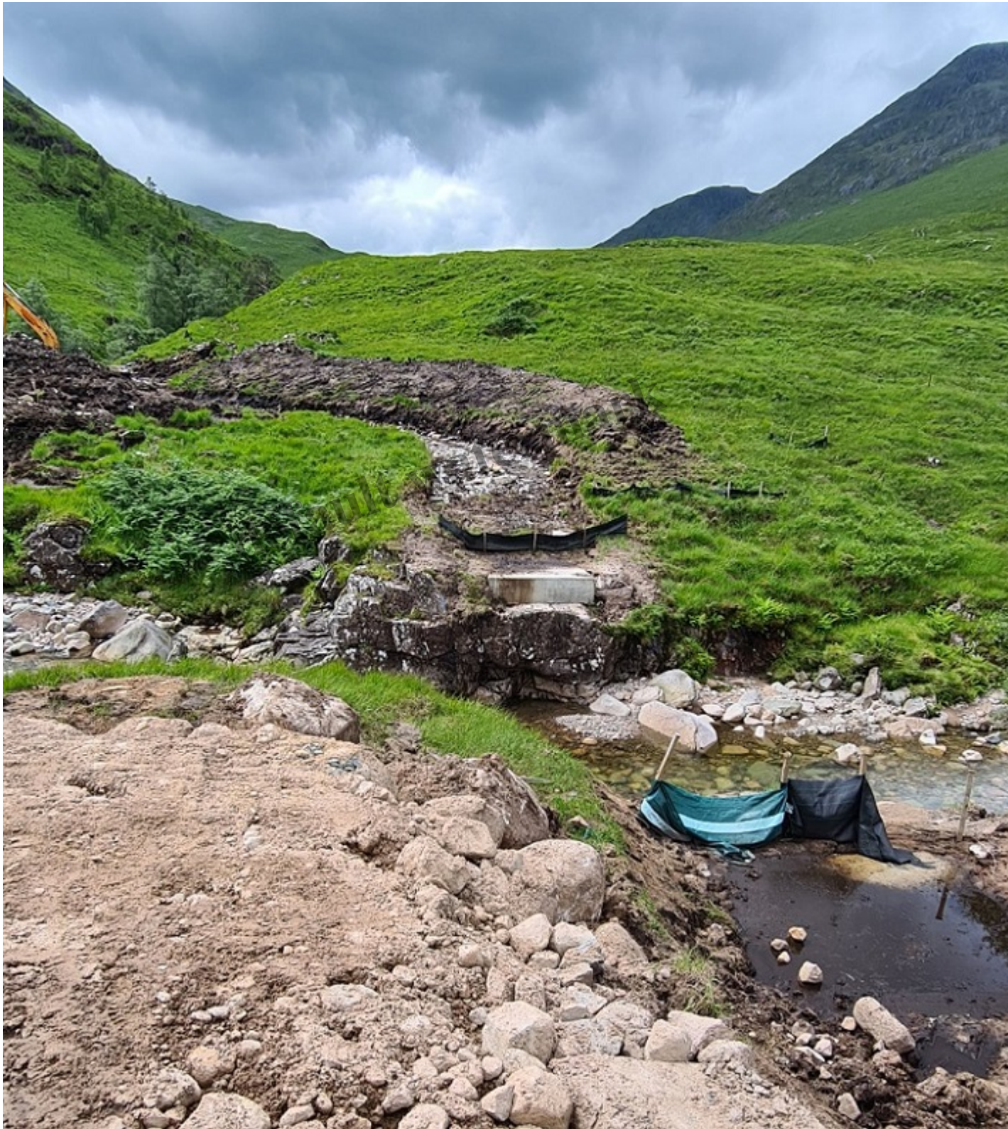
Construction track through peat to the intake with concrete foundation for bridge
