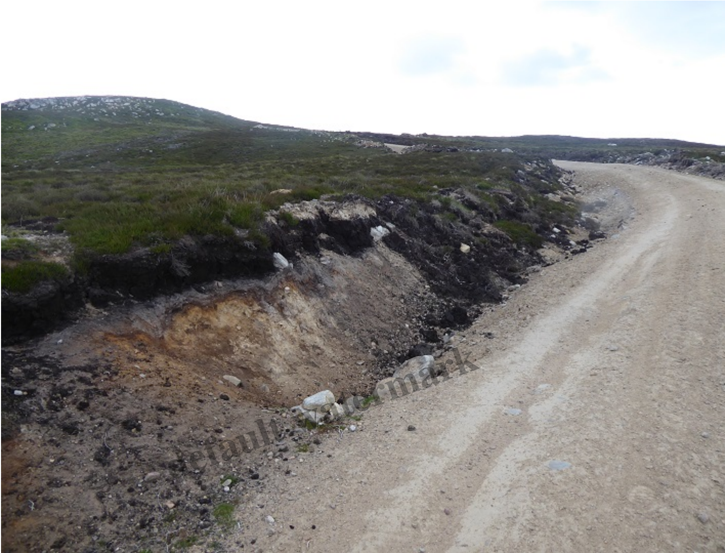
Section of edge of track that had been restored with vegetation above an unrestored section below
