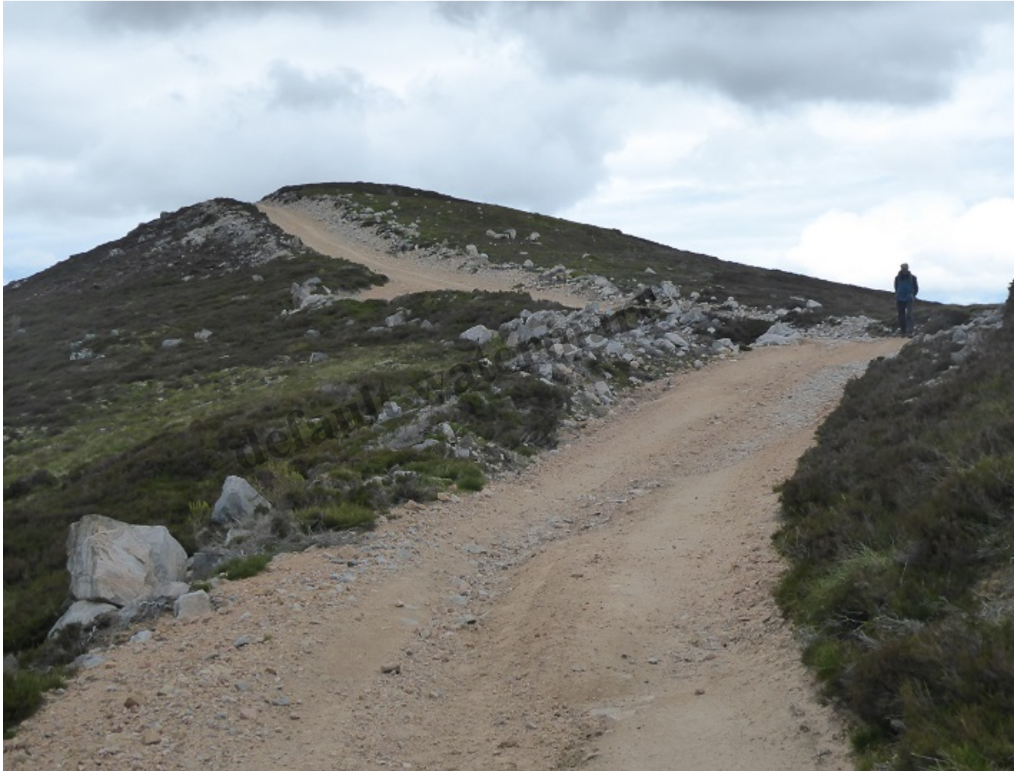
The upgraded road over the knoll north of Creag n'h Iolaire within the National park boundary
