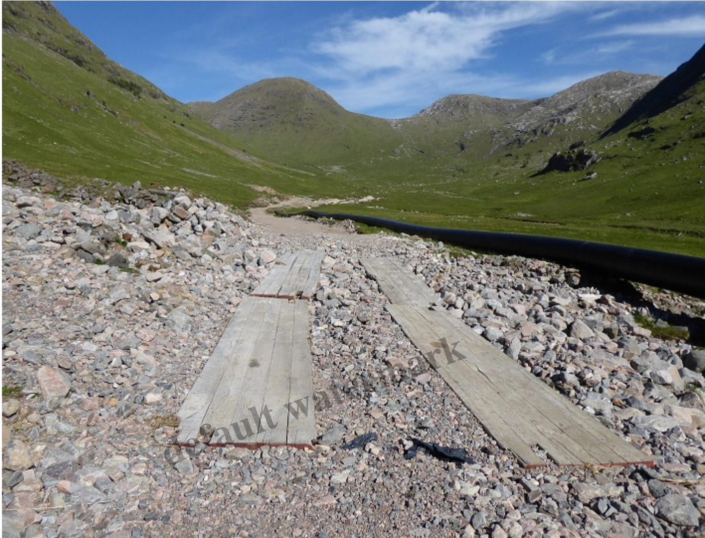
Pipeline by debris flow
