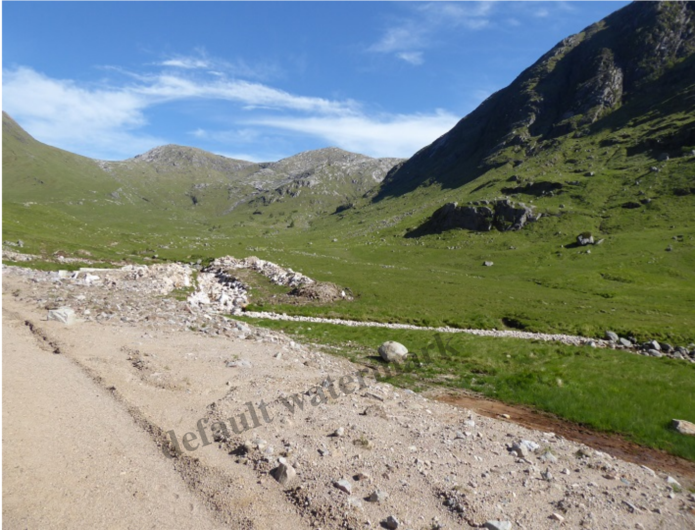
A little lower down is the transition between where the pipe was constructed through rocks and boulders and soil.
