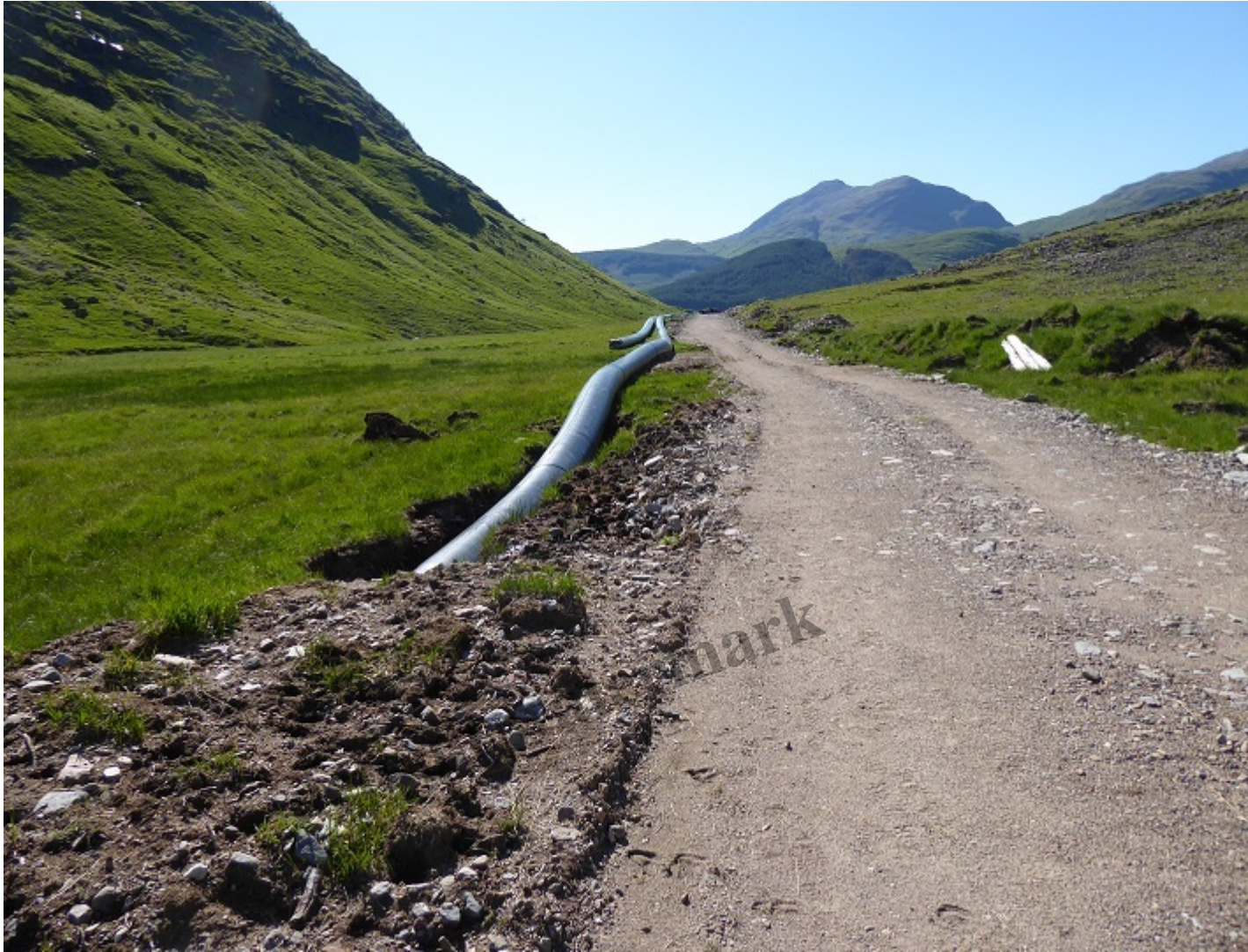
Looking down the grassy sward where the pipe is waiting to be buried
