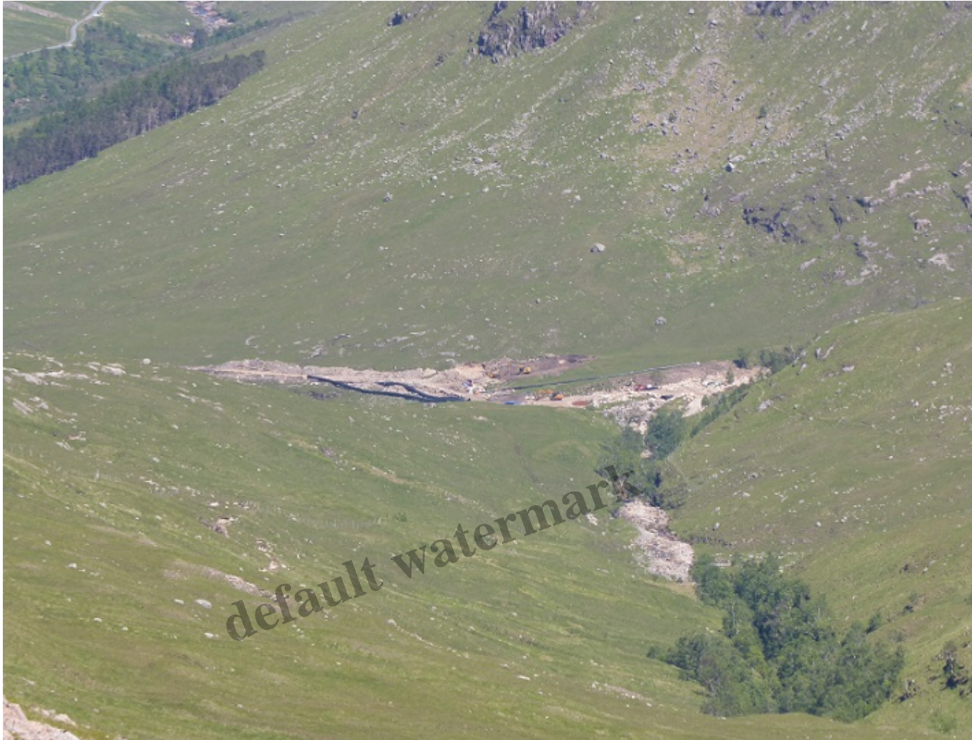
The Allt Chaorainn intake – note the vehicles and pipeline yet to be buried – and a section of the access track constructed through granite slabs viewed from the slopes of Beinn Ceitlein
