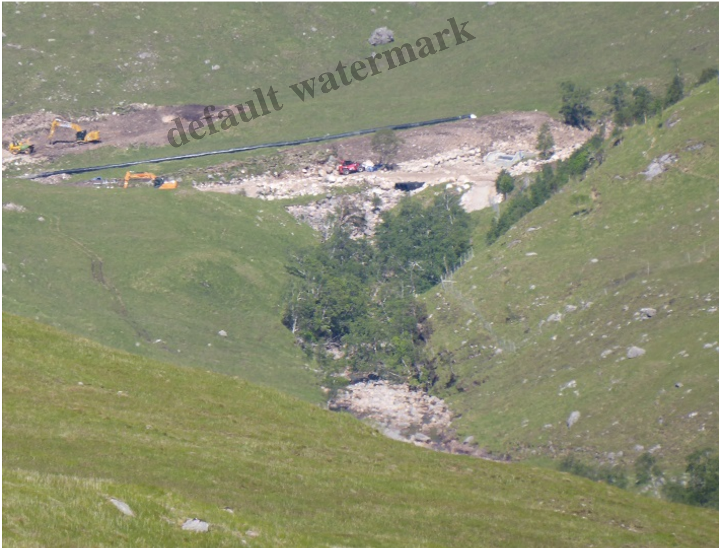
Work on the Allt Chaorainn intake and pipeline viewed from the east slopes of Beinn Ceitlein. Photo
