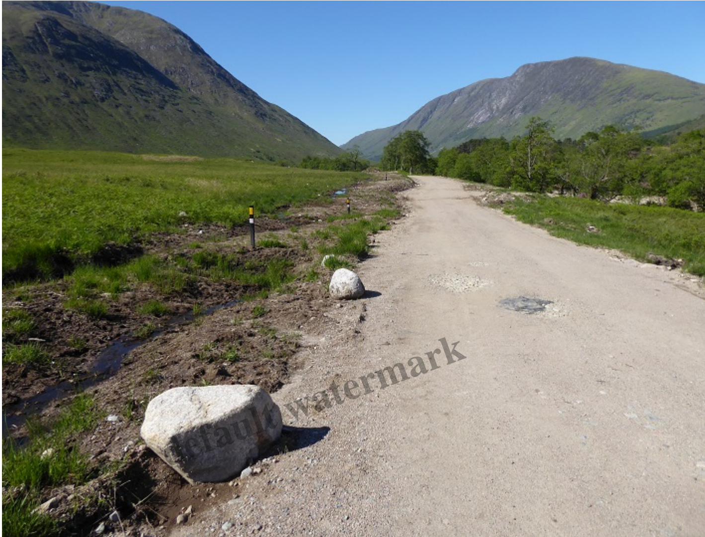
The new track to the Allt Mheuran power house (1 in top photo), in part “floated” over peat bog. The plastic poles on the left, an intrusion into a once wild landscape, mark a section of under-grounded power line.
