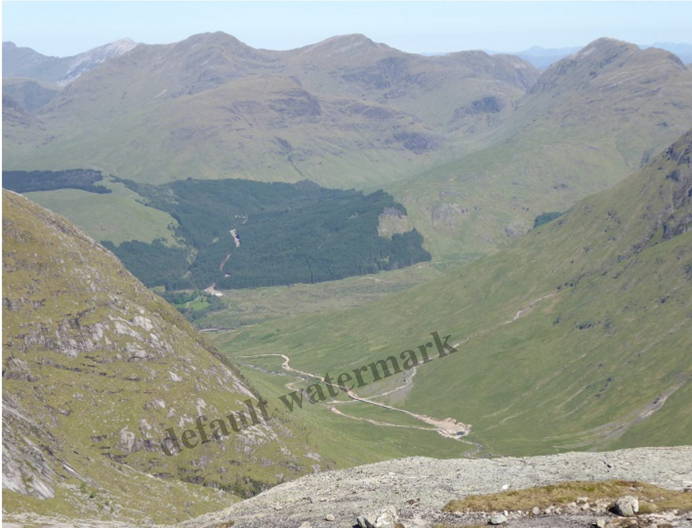
The Allt Ceitlein hydro, still under construction, with the Allt Charnan hydro scheme behind on the far side of Glen Etive viewed from Meall Tarsuinn
